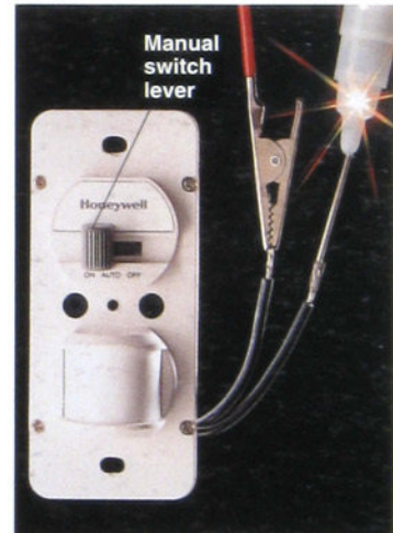
Motion-sensor switch: Attach the tester to a wire lead and touch the test probe to the
