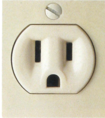
15 amps, 125 volts. Three-slot grounded receptacle has two different size slots and a U-shaped hole for grounding. It is required in all new wiring installations.
