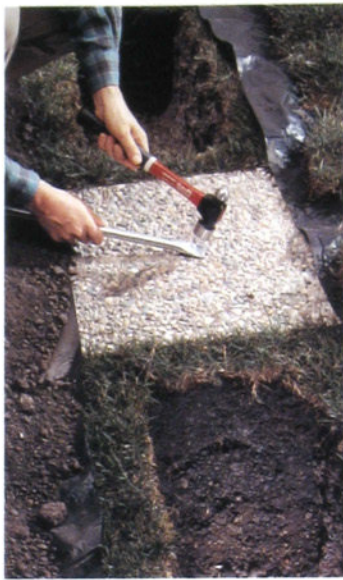
5 To run cable under a sidewalk, cut a length of metal conduit about 1 foot longer than the width of the sidewalk, then flatten one end of the conduit to form a sharp edge.
