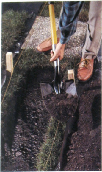
4 Dig 6 inches to the depth required by your local code. The second string line is used to mark the trench.
