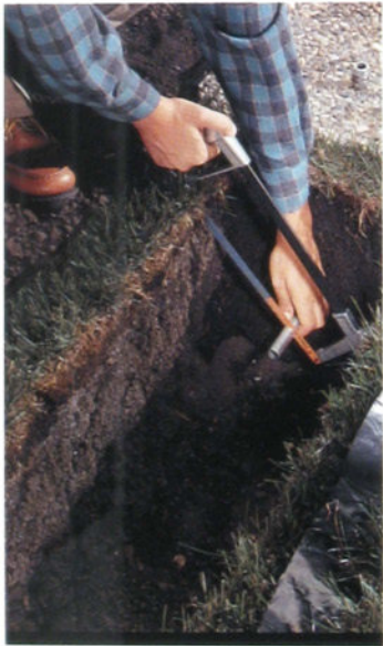
7 Cut off the ends of the conduit with a hacksaw, leaving about 2 inches of exposed conduit on each side. Underground cable will run through the conduit.
