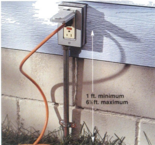
Prevent shock by making sure all outdoor recepta- protected by GFCIs (page 74). A single GFCI can be wired to protect other fixtures on Outdoor receptacles should be at least round level and enclosed in weather- boxes with watertight covers.
