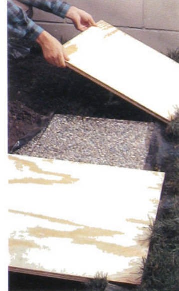
9 If trenches must be left unattended, temporarily cover them with scrap plywood to prevent accidents.
