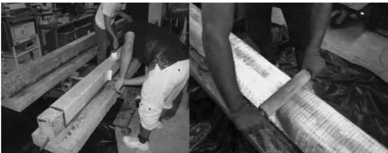
FIGURE 8.8 Applying resin to FRP with a paint roller (left) and clearing the air pockets with a wooden roller (right).
