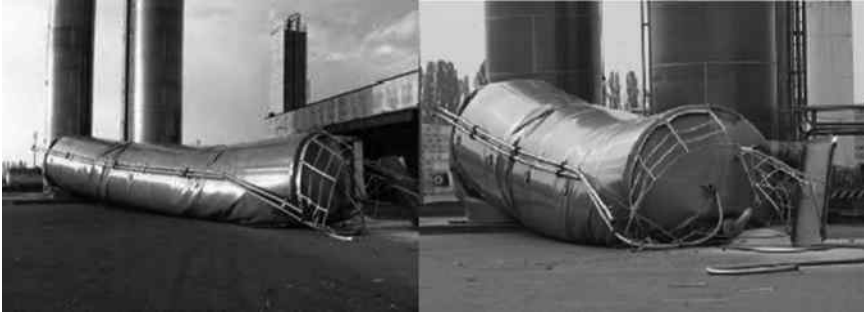
Figure 1.67 The collapse of a steel silo during the Emilia earthquake. (Faggiano, B. et al. 2012: Steel buildings within the Emilia earthquake (in Italian). Progettazione Sismica , n.3, IUSS Press, ISSN 1973–7432.)
