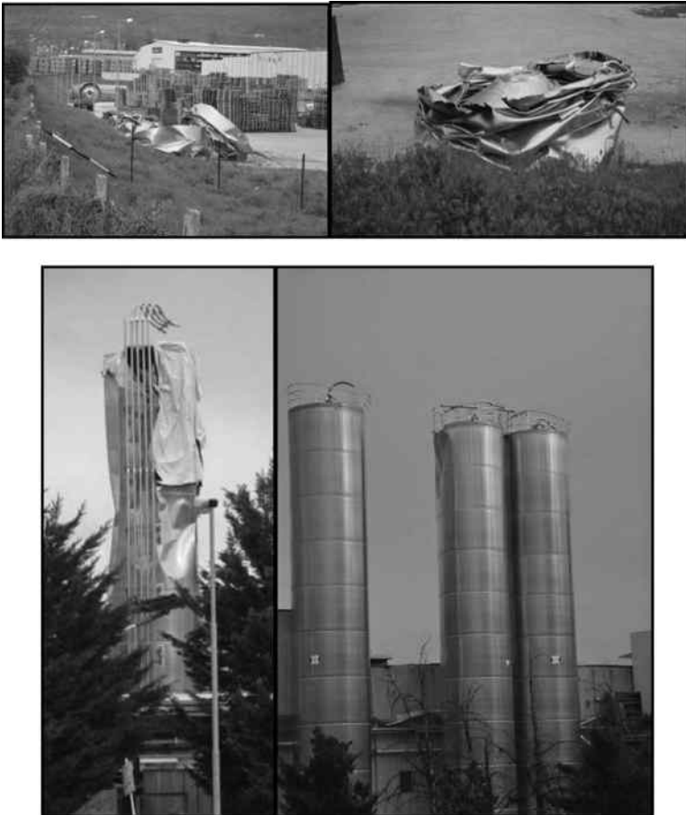
Figure 1.64 Local and global failure of silos.
