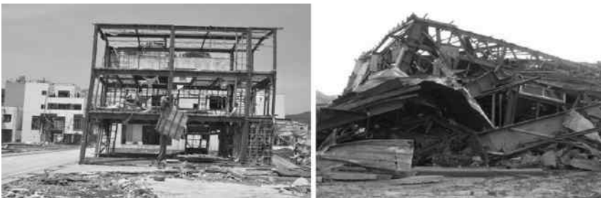
Figure 1.55 Structure damage and collapse due to tsunami. (After Midorikawa M. et al. 2012: Earthquake and tsunami damage on steel buildings caused by the 2011 Tohoku Japan earthquake. International Symposium on Engineering Lessons Learned from the 2011 Great East Japan Earthquake , Tokyo, March 1–4, 1061–1076.)
