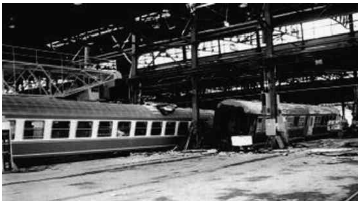
Figure 1.43 Damaged steel building of the railcar factory. (After Erdik, M. 2000: Report on 1999 Kocaeli (Turkey) Earthquake. Bogazici University Report 2000.)
