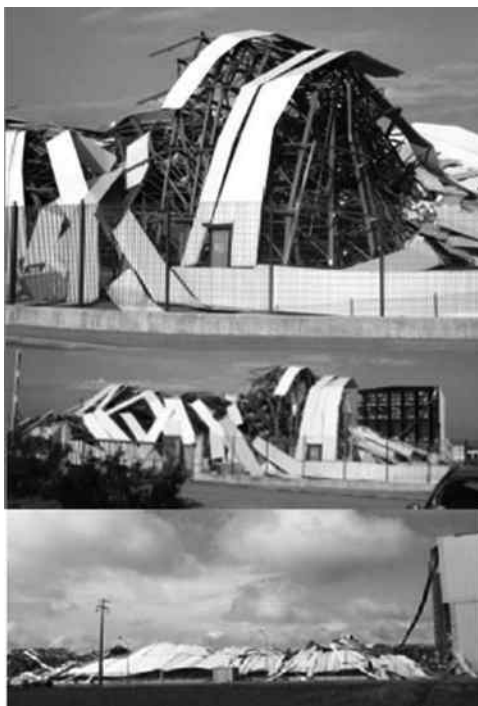
Figure 1.66 The collapse of an industrial building during the Emilia earthquake. (Faggiano, B. et al. 2012: Steel buildings within the Emilia earthquake (in Italian). Progettazione Sismica , n.3, IUSS Press, ISSN 1973–7432.)
