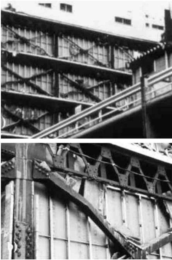
Figure 1.29 Buckling of bracings. (Gioncu, V., Mazzolani, F.M. 2002: Ductility of Seismic Resistant Steel Structures . Spon Press, London; after Fischinger, M. 1997: EASY, Earthquake Engineering Slide Information System. FGG-IKPIP Institute Slovenia.)
