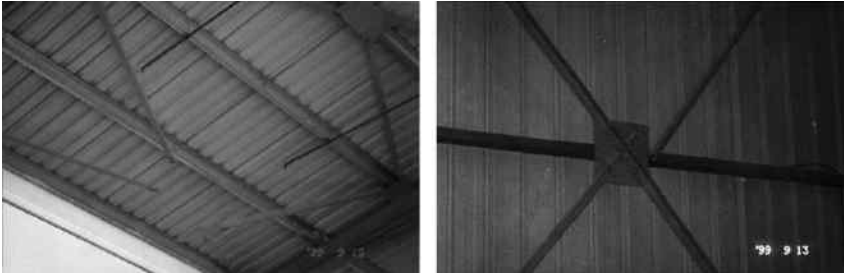
Figure 1.62 Bracing fractures during the 1999 Athens earthquake. (Altay, G. 2005: Post-earthquake damage assessment in the Mediterranean regions. Earthquake protection of historical buildings by reversible mixed technologies, PROHITECH, WP 2.)
