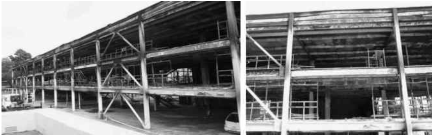
Figure 6.11 The steel building of the University of Chile damaged by fire after an earthquake. (Photo by Mazzolani.)
