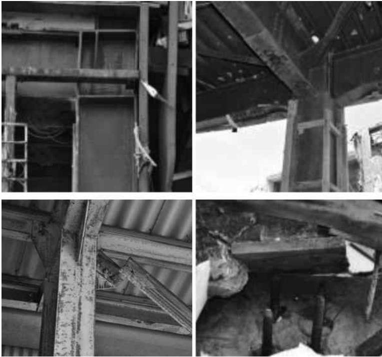
Figure 1.54 Damage or fractures of connections, braces, and anchor bolts due to ground motions. (After Midorikawa M. et al. 2012: Earthquake and tsunami damage on steel buildings caused by the 2011 Tohoku Japan earthquake. International Symposium on Engineering Lessons Learned from the 2011 Great East Japan Earthquake , Tokyo, March 1–4, 1061–1076.)
