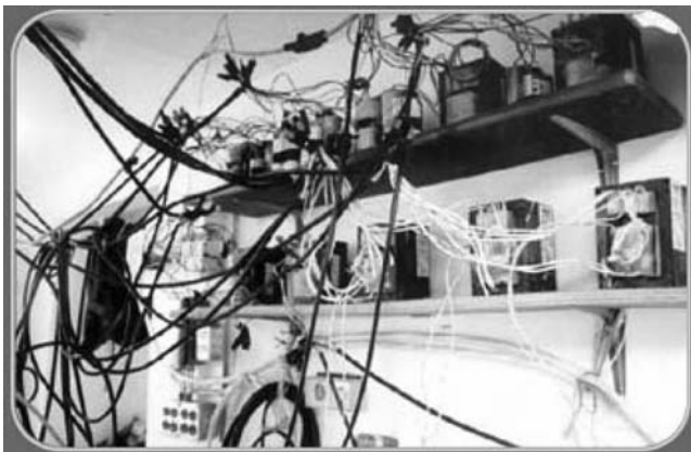
Figure 9.1 Example of a non-conforming electrical installation! (courtesy StingRay)
