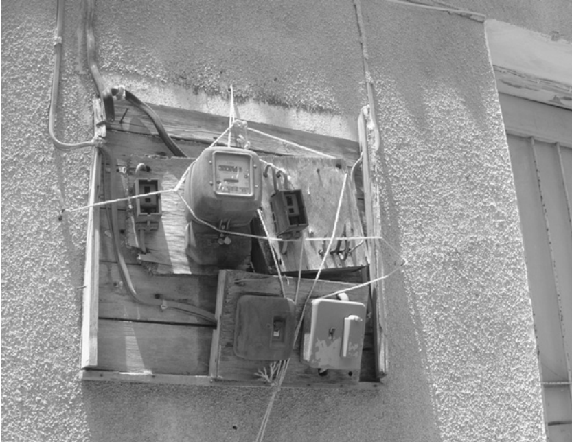
Figure 6.4 Certainly NOT the right sort of installation! (courtesy of StingRay)
