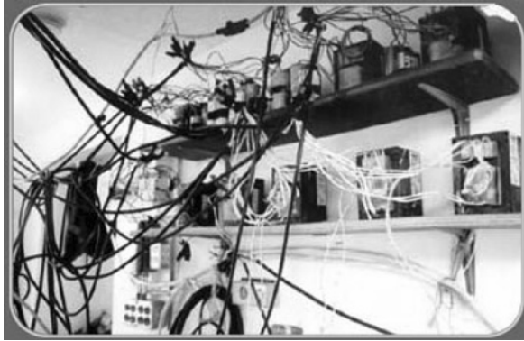
Figure 9.2 Example of a non-conforming electrical installation!
