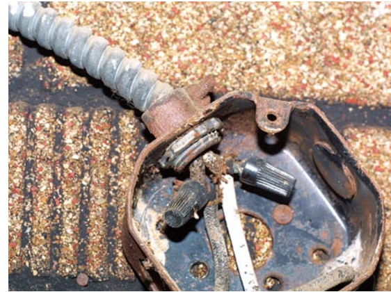
Armored cable terminates in an outlet box in a 1930s home.
