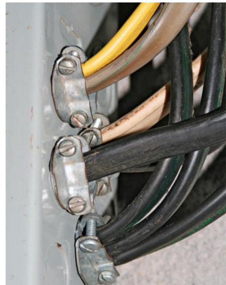
NM clamps tightening on the side of cable can damage the cable (top). A singular clamp if overtightened can damage cable (extremely common) (middle). Three cables (against code) in a NM clamp almost guarantees a damaged cable (bottom).
