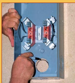
66 | Locating the Meter Base
