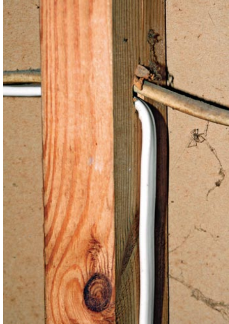
Pinch point. Never pull an immediate turn with a cable. It can heat up and arc.
