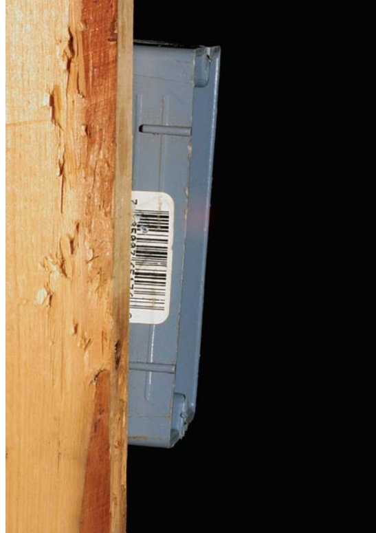
The front edge of the box must be parallel with the stud—not angled like the one shown here—extending just far enough to make it flush with the finished wall.
