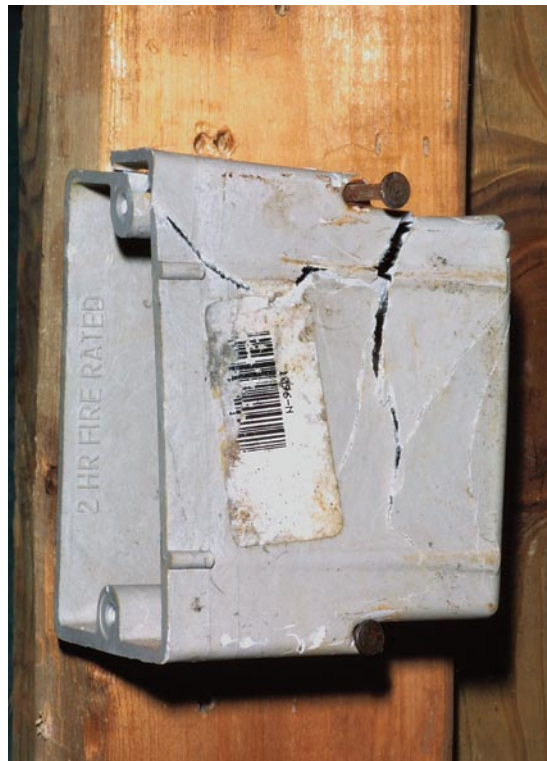
Fiberglass boxes are sturdy but can easily be destroyed by one misplaced hammer blow.
