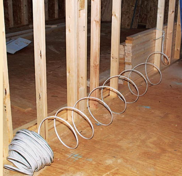
Letting the cable spin out will leave it in spirals—making it impossible to pull it through the studs.
