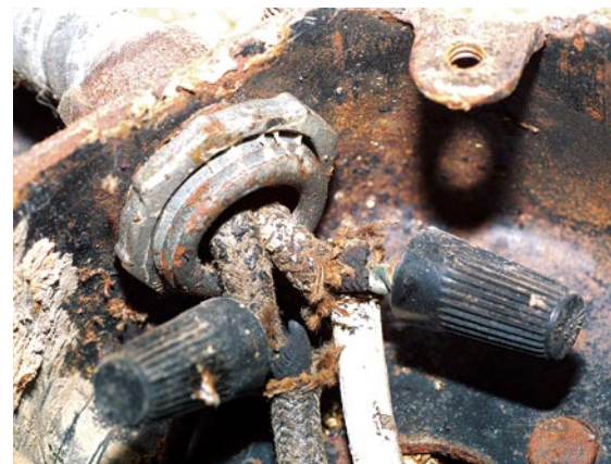
Even close up you can just barely differentiate the black (hot) from the white (neutral) conductor. The insulation on both wires is severely deteriorated and may break away if the wires are moved.
