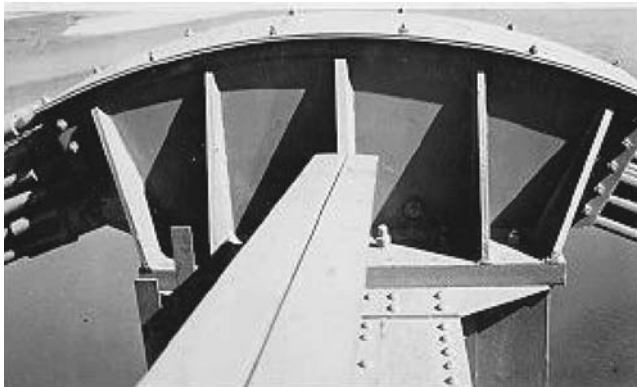
Fig. 8.6 The top of the towers, where the main cable passes over the saddle, transferring the load down vertically into the tower leg. ( www.inventionfactory.com/history/RHAbbridg/term/ )
