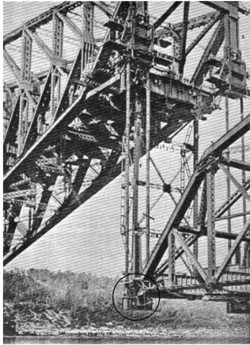
Fig. 4.25 A close-up of the hanger arm and one of the corner bearings. (Hammond: Engineering Structural Failures – the causes and results of failure in modern structures of various types)
