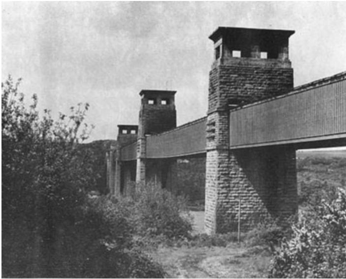
Fig. 13.15 The sagging of the bridge spans because of the vertical split over the intermediate supports. ( http://vivovoco.rsl.ru/MV/E_LESSON/BRIDGES/BRIT/BRIT.HTM )
