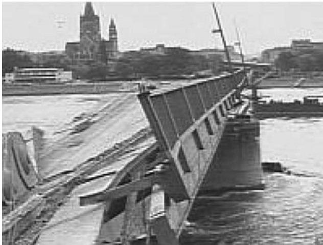
Fig. 18.6 The end span supported by the collapsed river pier (to the bottom right in Fig. 18.5 above). ( www.reichsbruecke.net/geschichte_e.php )
