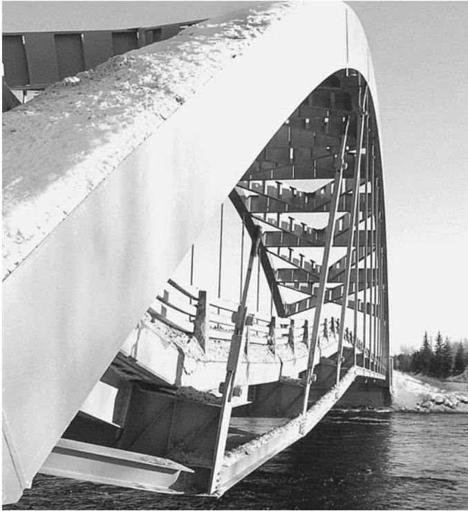
Fig. 20.15 The (partial) collapse of the Sgt. Aubrey Cosens VC Memorial Bridge. ( http://speaker.northernontario.ca/content/Feature%20Story/C%20Front%2011:01:06.pdf )
