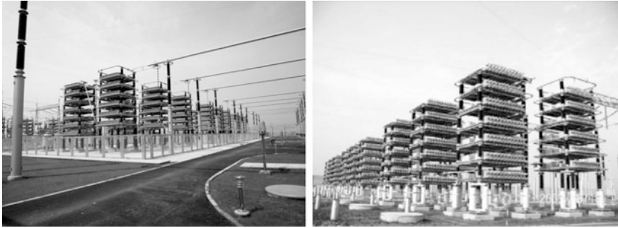
Fig. 26.10 Installed AC filters and shunt capacitors
