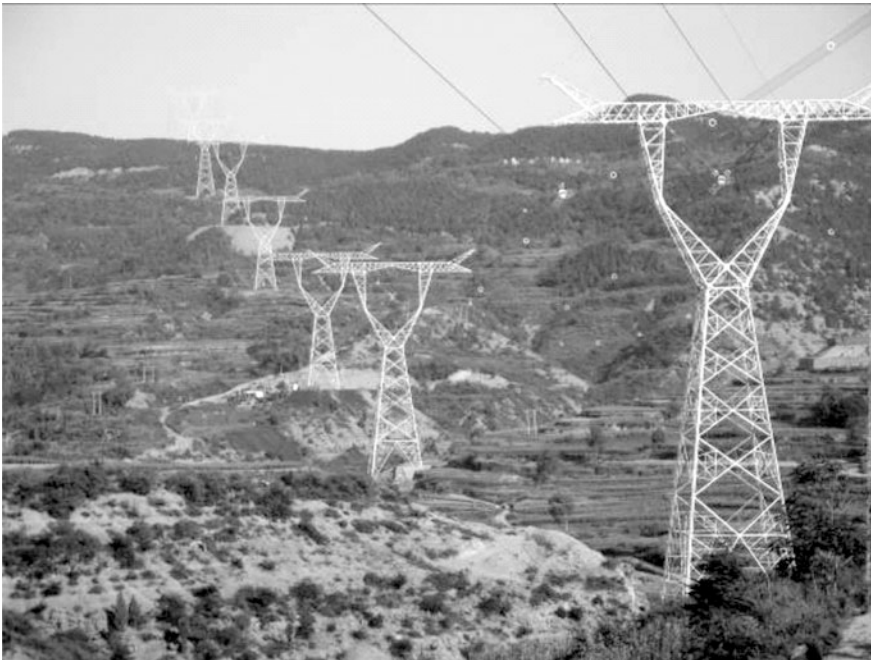
Fig. 27.1 Southeast Shanxi-Nanyang-Jingmen 1000 kV UHVAC single-circuit transmission line
