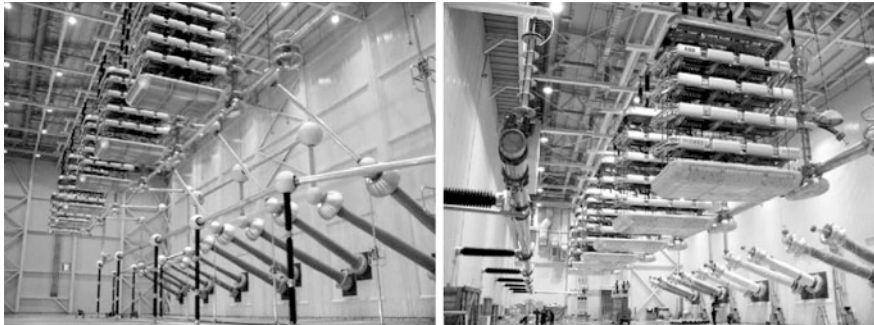
Fig. 26.7 Completed converter valves
