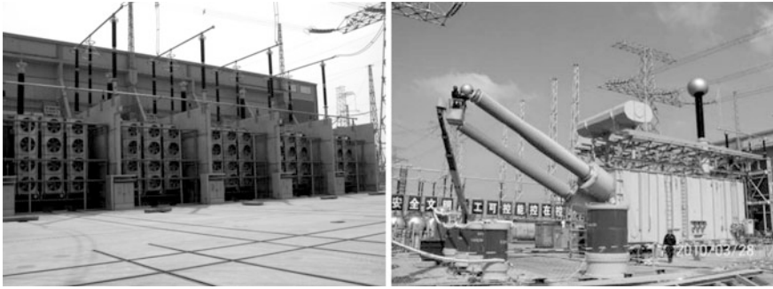
Fig. 26.8 Converter transformers that are installed and being installed
