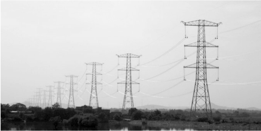
Fig. 27.2 Huainan-South Anhui-North Zhejiang-West Shanghai 1000 kV UHVAC double-circuit transmission line
