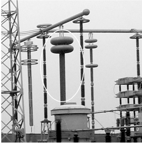
Fig. 21.23 Pole line voltage measuring equipment in Fulong Station of Xiangjiaba-Shanghai \pm 800 kV UHVDC transmission project
