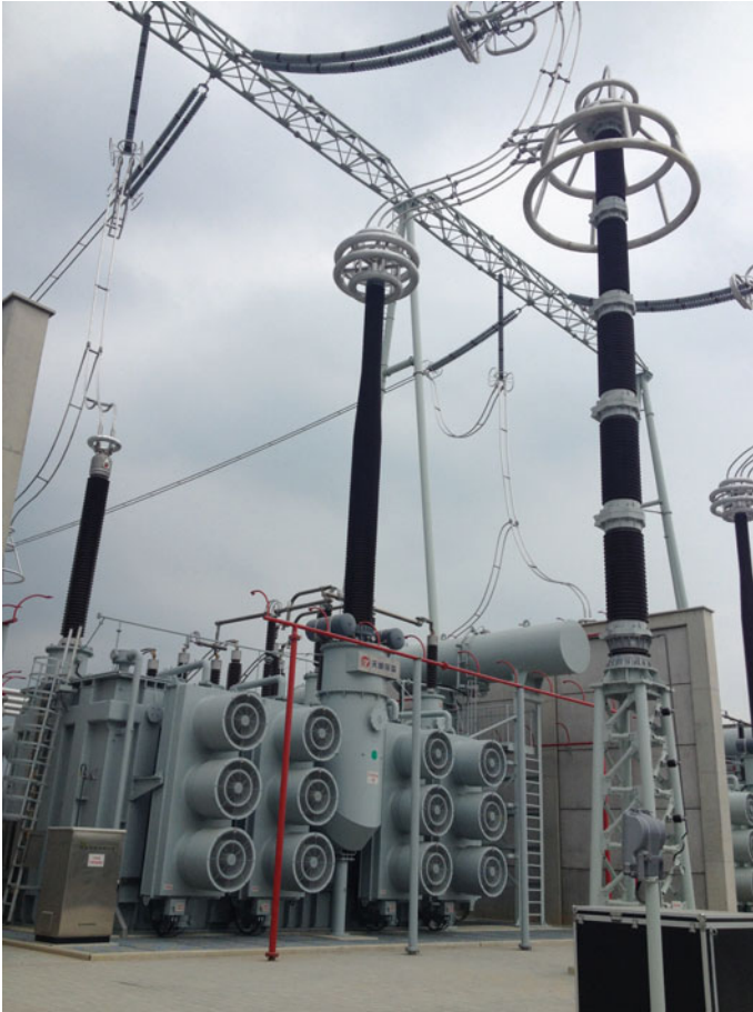
Fig. 25.3 Photo of 1000 kV main transformer
