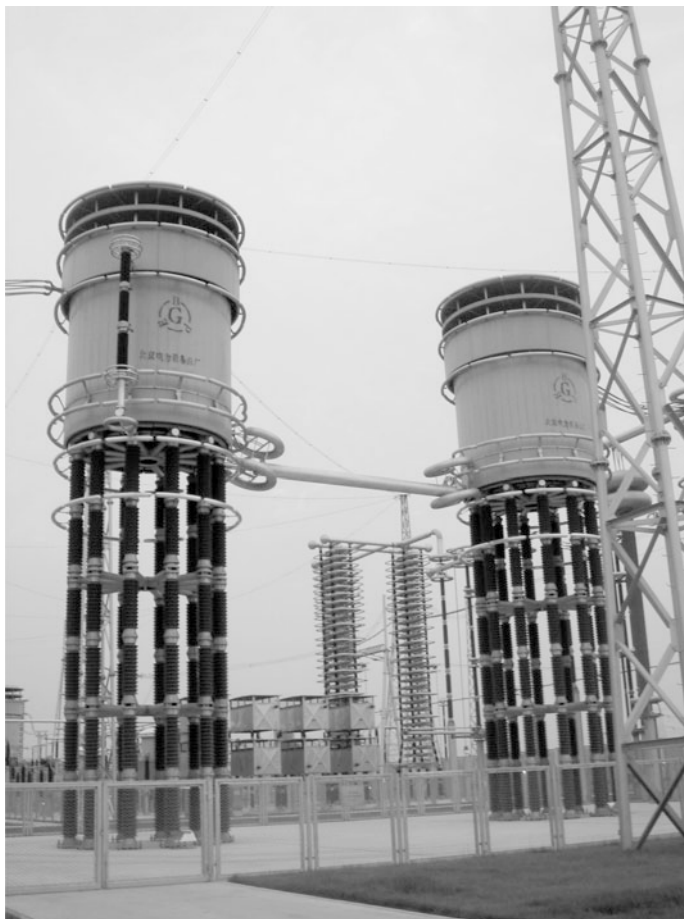
Fig. 21.9 Dry-type smoothing reactors in Fengxian Station of Xiangjiaba-Shanghai \pm 800 kV DC project
