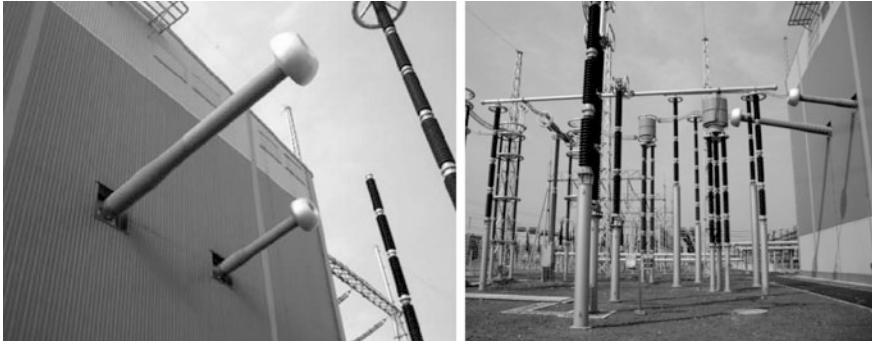
Fig. 26.13 Installed wall bushing
