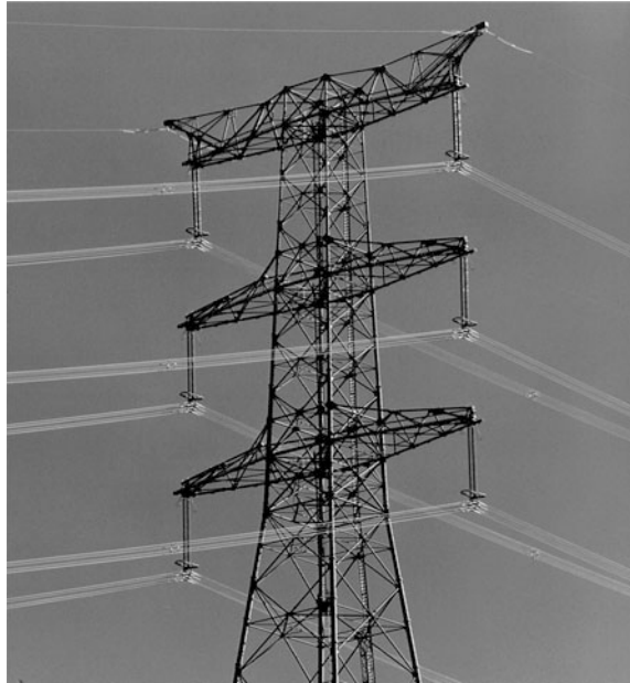
Fig. 1.3 UHV transmission lines in Japan
