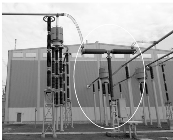
Fig. 21.22 Bypass switch of LV valve in Fulong Station of Xiangjiaba-Shanghai \pm 800 kV UHVDC transmission project
