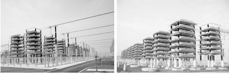
Fig. 21.10 Installed AC filters
