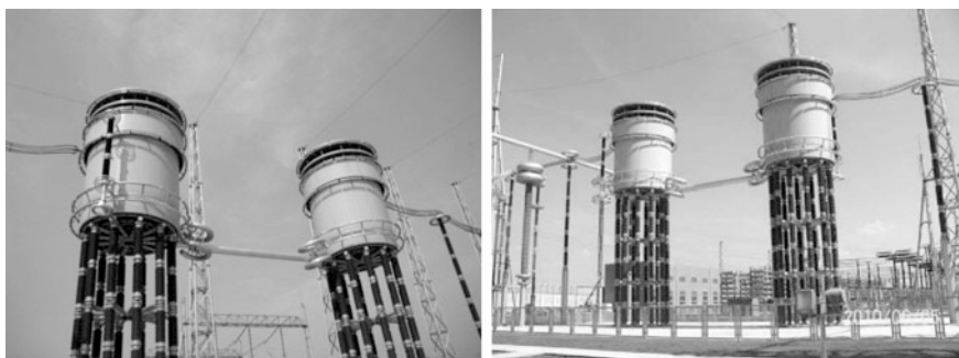
Fig. 26.9 Installed smoothing reactor
