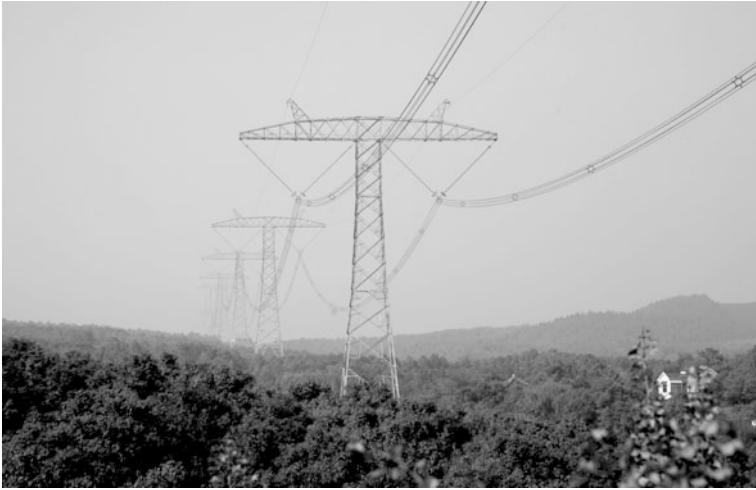
Fig. 28.1 \pm 800 kV Xiangjiaba–Shanghai UHVDC transmission line
