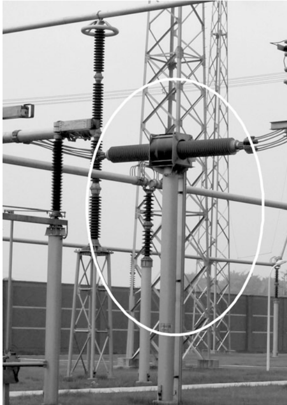
Fig. 21.24 Current transformer on neutral line in Fulong Station of Xiangjiaba-Shanghai \pm 800 kV UHVDC transmission project
