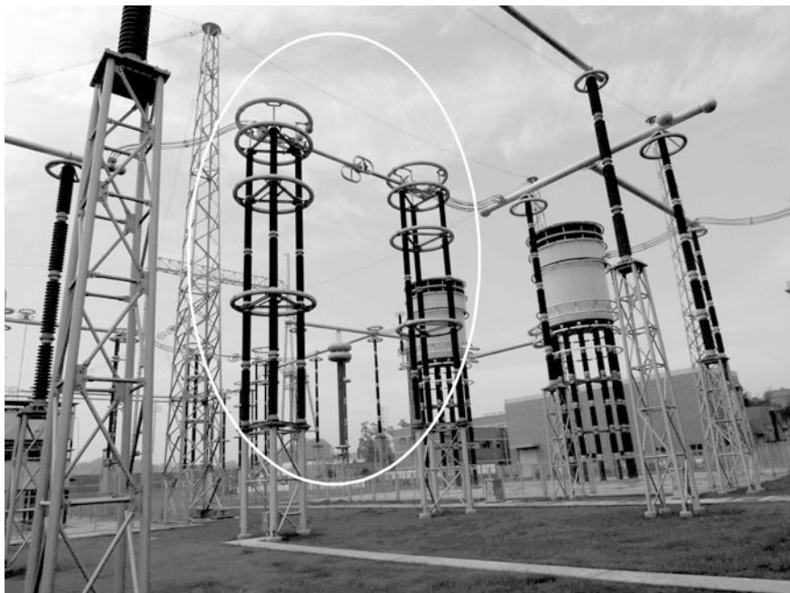
Fig. 21.21 Disconnectors on neutral line in Fulong Station of Xiangjiaba-Shanghai \pm 800 kV UHVDC transmission project
