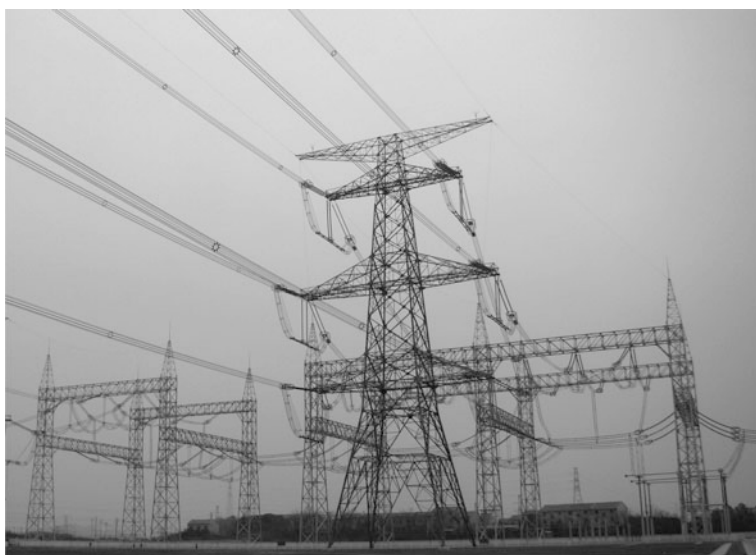
Fig. 2.5 Double-circuit test lines
