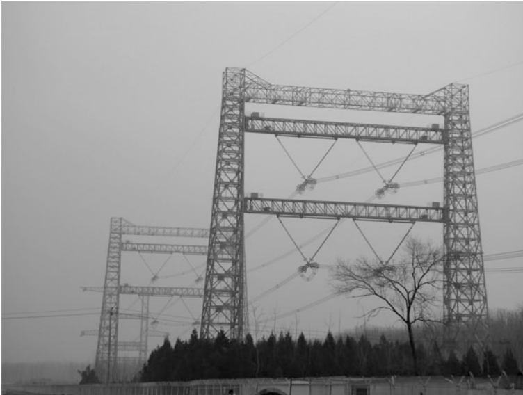
Fig. 2.6 UHVDC test lines and towers
