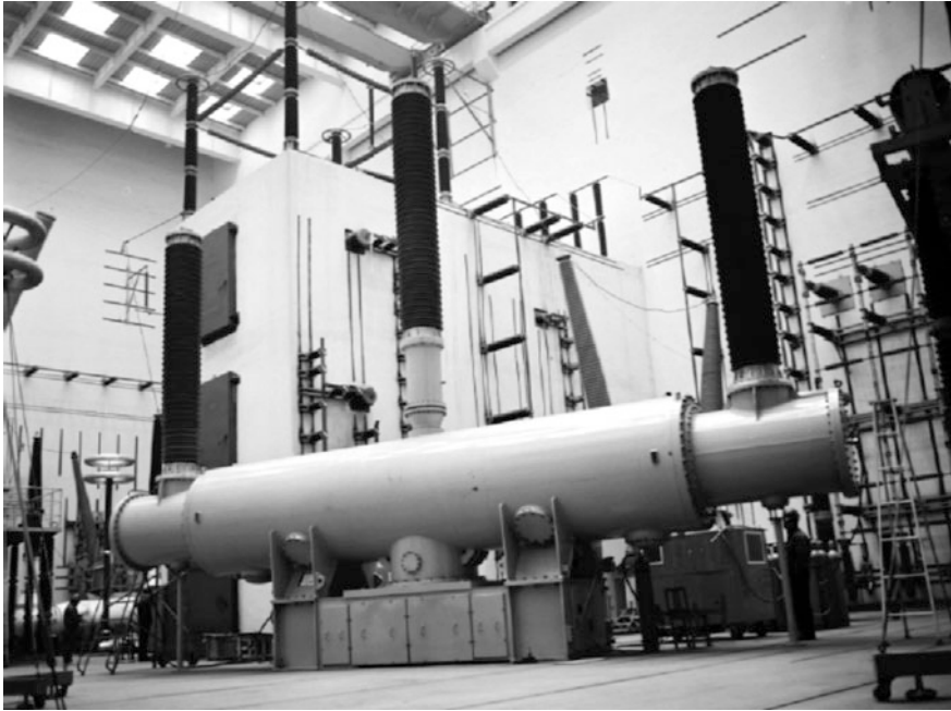
Fig. 11.16 UHV GIS equipment
