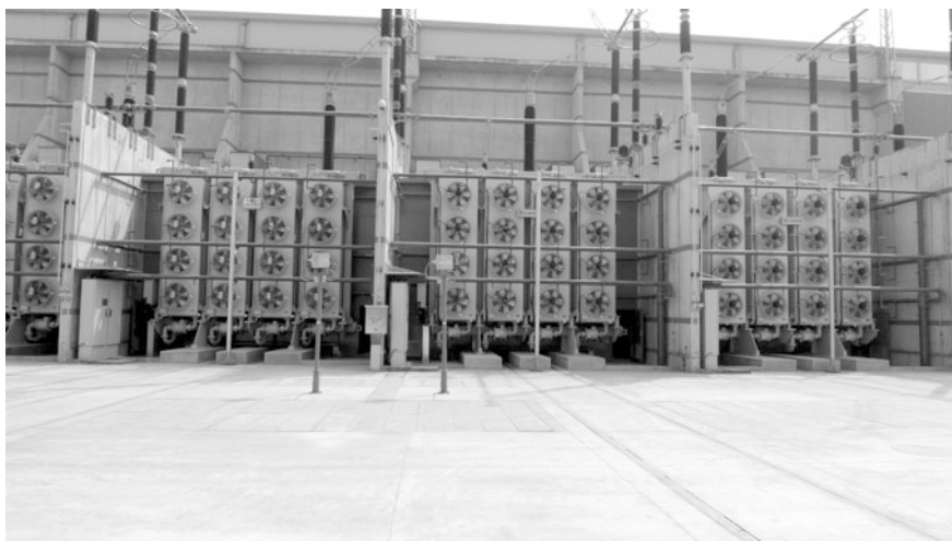
Fig. 21.3 Arrangement of converter transformers outside valve hall
