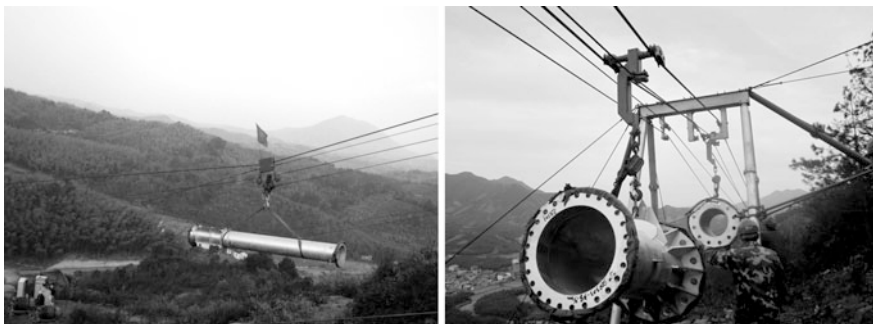
Fig. 27.21 Transportation of steel tubes by ropeways for the lines located in the Hilly areas
