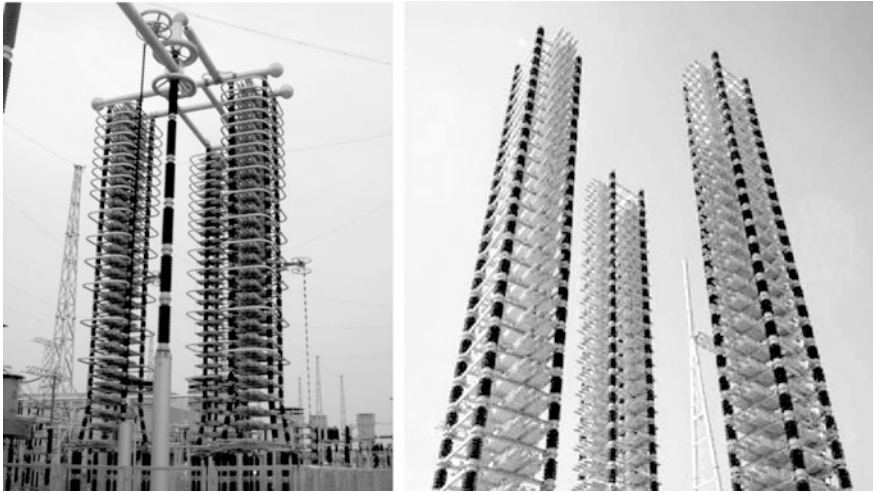
Fig. 21.11 Installed DC filter banks
