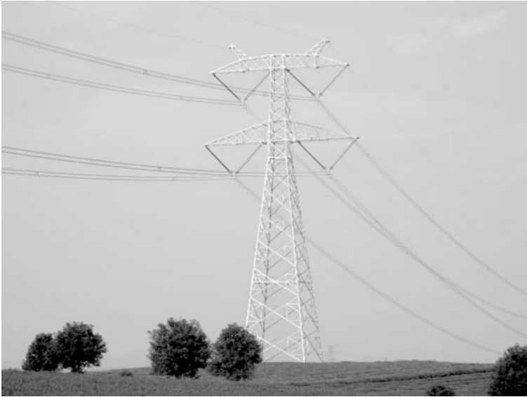
Fig. 28.11 Double-circuit DC line of \pm 500 kV Jinmen–Fengjing Project
