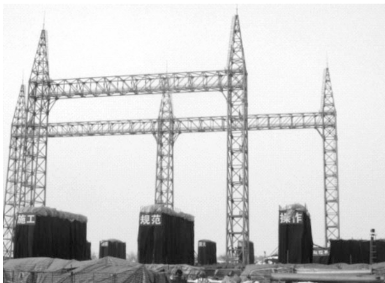
Fig. 25.14 1000 kV lattice framework of Southeast Shanxi substation
