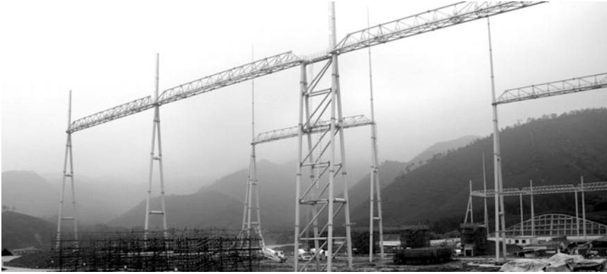
Fig. 25.15 1000 kV herringbone column framework of North Zhejiang substation
