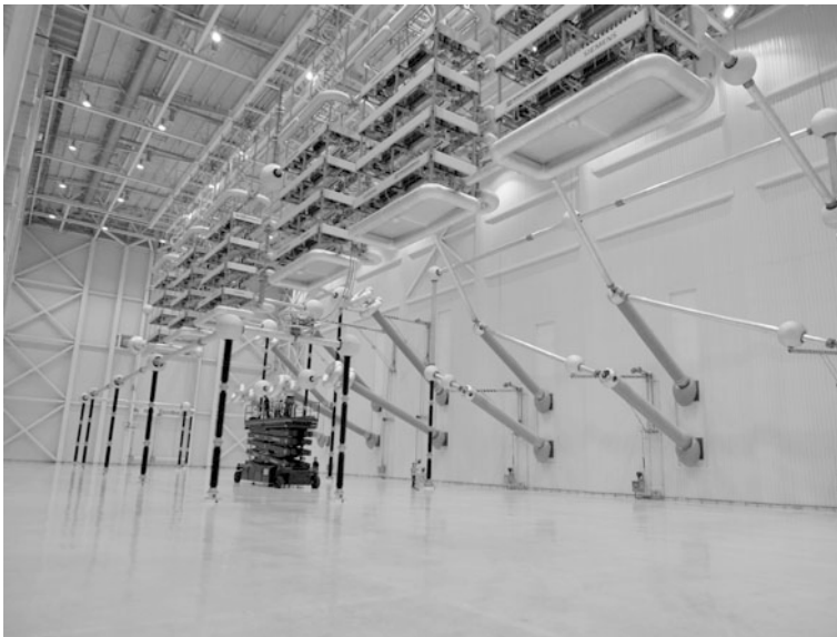
Fig. 21.7 Suspended converter valve used in Fulong Station
