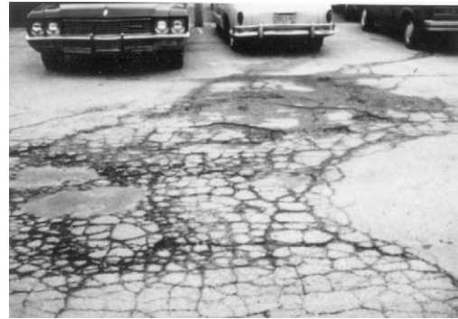
FIGURE 8.16 Alligator cracking developed due to cycles of freeze and thaw combined with poor drainage.
