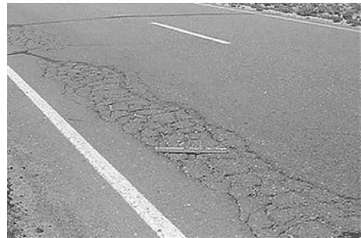
FIGURE 8.5 Advanced stage of fatigue cracking.
