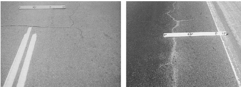
FIGURE 19.15 Meandering cracks in flexible pavements (Source: Austroads, 1987).
