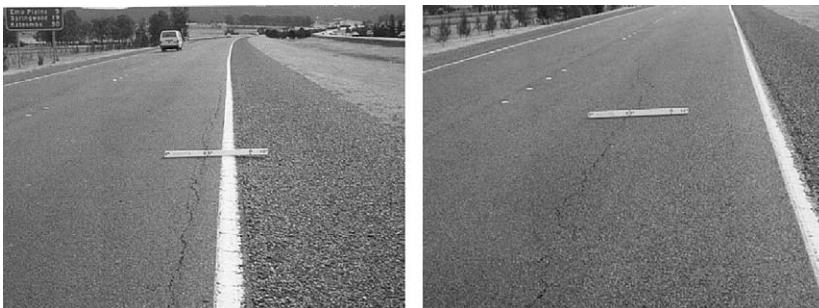
FIGURE 19.10 Longitudinal cracks in flexible pavements (Source: Austroads, 1987).
