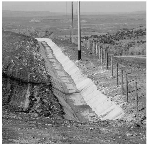
FIGURE 13.6 Concrete linked ditch.
