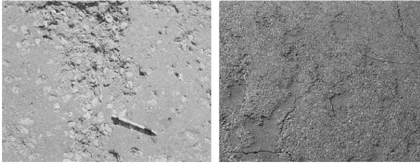
FIGURE 19.20 Raveling in flexible pavements (Source: Austroads, 1987).
