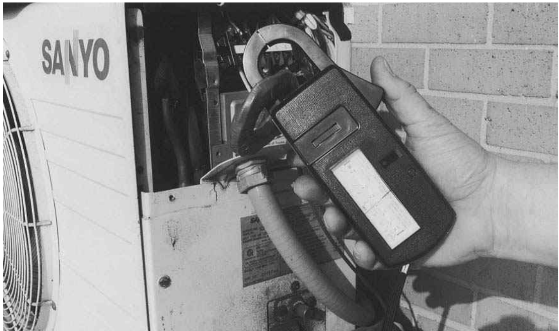
Figure 1-26 A scale divider and clamp-on ammeter being used to measure the control current in an air conditioner.
