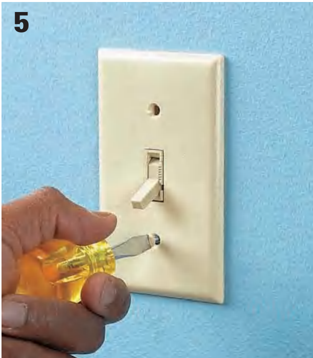
5 Attach the cover plate to the new wireless switch. Turn the power service back on, and test to make sure the switch operates normally.
