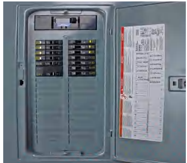
Create a circuit index and affix it to the inside of the door to your main service panel. Update it as needed.
