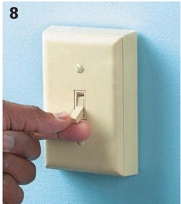
8 Test the operation of both switches. Each switch should successfully turn the light fixture on and off. You've just successfully created a three-way switch installation without running any new wires.
