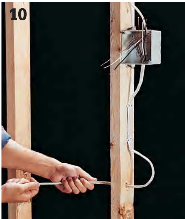
10 Continue the circuit by running cable between each pair of electrical boxes, leaving an extra 1 ft. of cable at each end.
