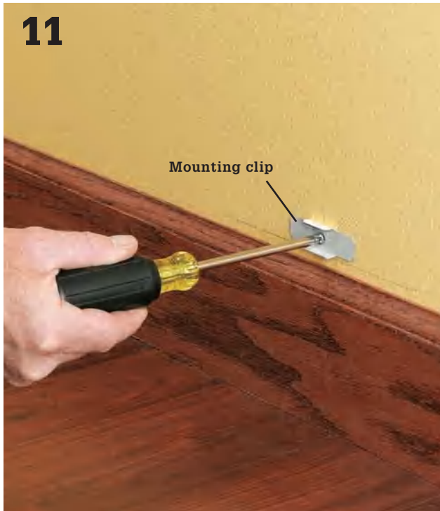
11 At stud locations mark a reference line \frac{1}{4} " above the top of the baseboard. Attach mounting clips for the track at these marks.
