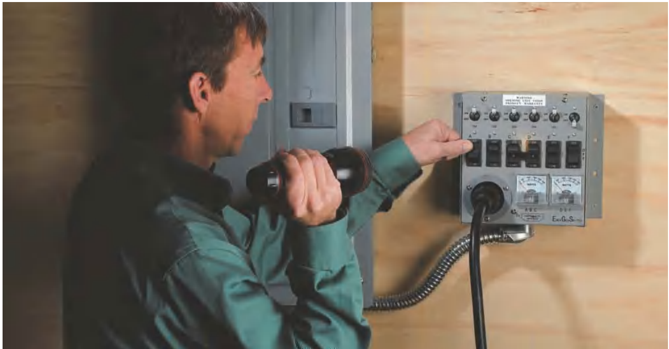
One flip of a switch reassigns the power source for each critical circuit so your backup generator can keep your refrigerator, freezer, and important lights running during an outage of utility power.
