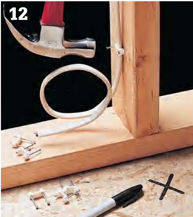
12 For a surface-mounted fixture such as a baseboard heater or fluorescent light fixture, staple the cable to a stud near the fixture location, leaving plenty of excess cable. Mark the floor so the cable will be easy to find after the walls are finished.
