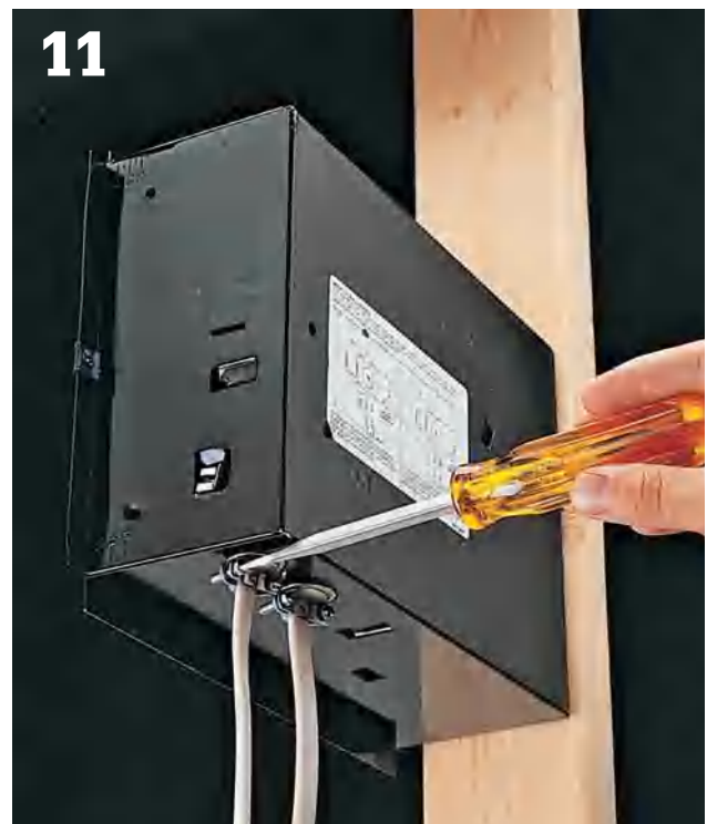
11 At metal boxes and recessed fixtures, open knockouts, and attach cables with cable clamps. From inside the fixture, strip away all but \frac{1}{4} " of sheathing. Clip back wires so there is 8" of workable length, and then strip \frac{3}{4} " of insulation from each wire.
