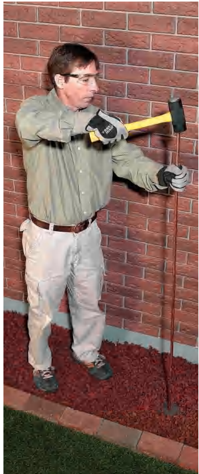
A pair of 8-ft.-long metal ground rods are driven into the earth next to your house to provide a path to ground for your home wiring system.
