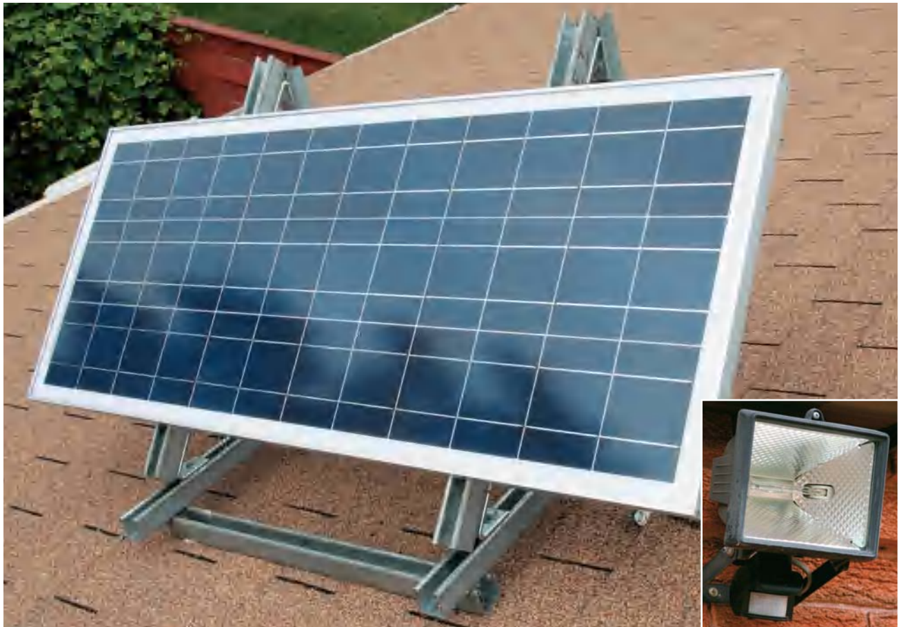
This 60-watt solar panel is mounted on a garage roof and powers a self-contained home security lighting system. Not only does this save energy costs, it keeps the security lights working even during power outages.
