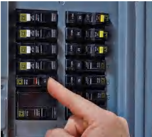
Shut power OFF at the main service panel or the main fuse box before beginning any work.
