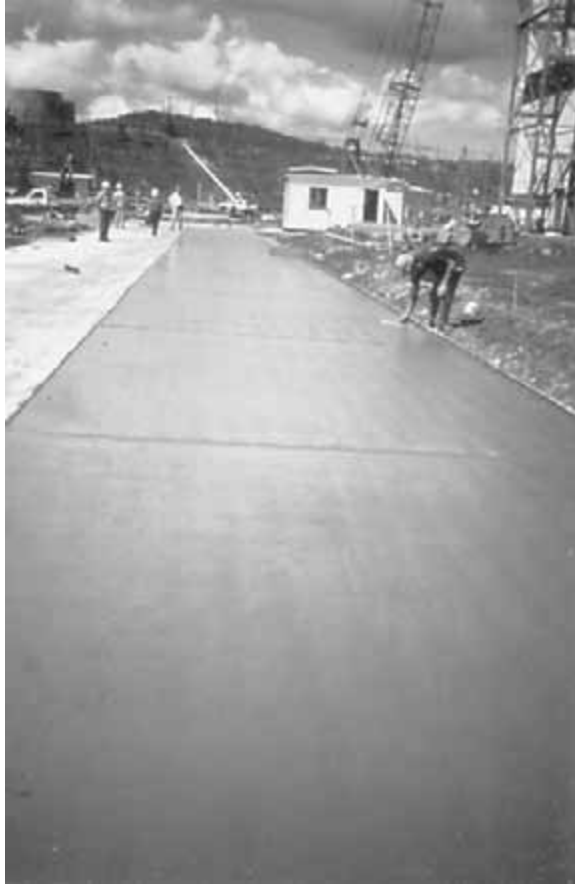
FIGURE 43.25 First pour of 32 MPa HVFA concrete in an apron slab at Mount Piper Power Station in New South Wales in 1991.
