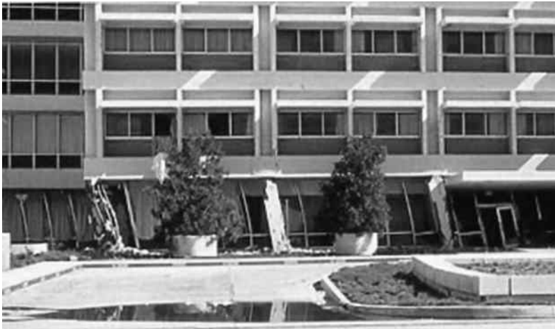
FIGURE 3.40 Olive View Hospital, San Fernando earthquake, 1971. Note the extreme deformation of the columns above the plaza level. (From FEMA-454, Designing for Earthquakes: A Manual for Architects . Washington, DC: Federal Emergency Management Agency, 2006.)
