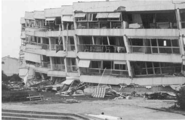
Collapse of frame concrete structures due to an earthquake. Courtesy of Murat Saatcioglu and John Gardner.
