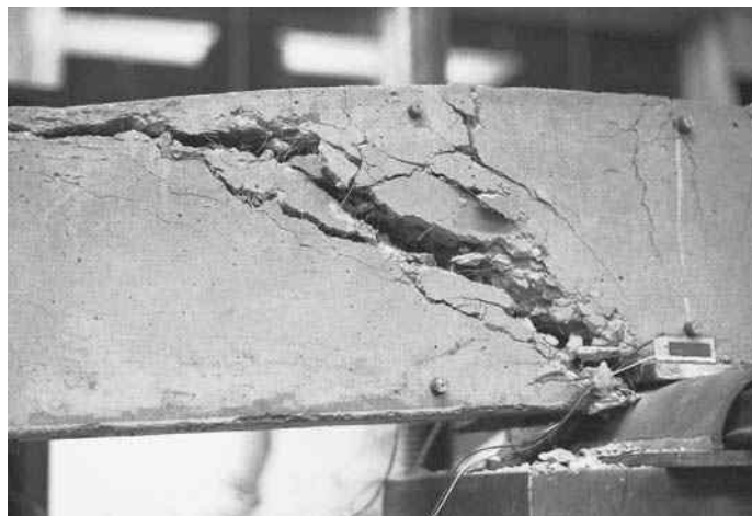
Shear failure near a middle support.
