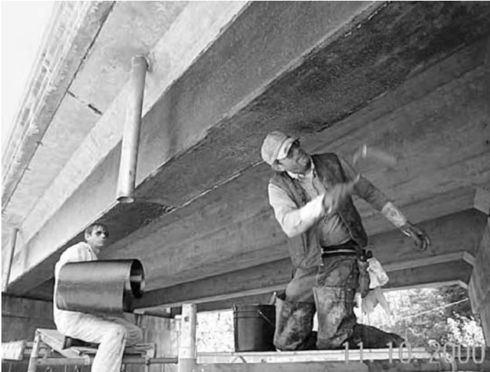
FIGURE 5.13 Preparations for wrapping the beam bottom with CFRP fabrics (Muddy Creek Bridge, West Virginia).
