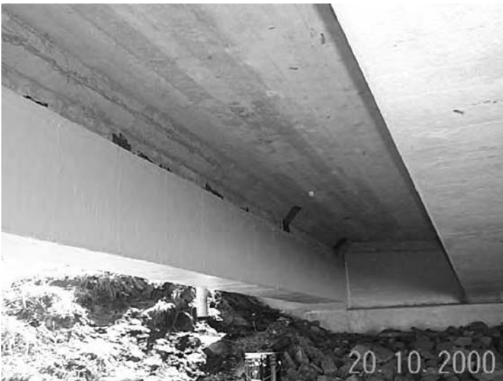
FIGURE 5.16 Finished interior of the external beam with carbon fabric and protective coating (Muddy Creek Bridge, West Virginia).
