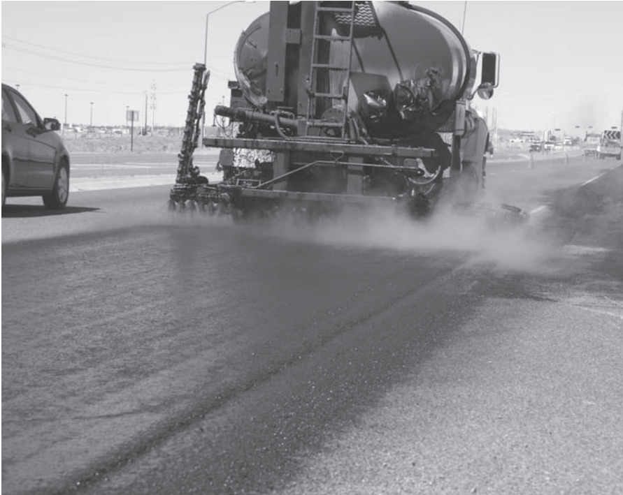
FIGURE 9.8 Spraying tack coat (emulsion) on existing asphalt pavement before placing an asphalt overlay. (Courtesy of FHWA)
