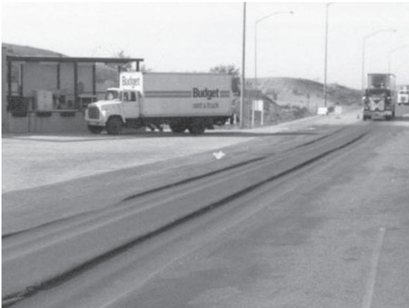
FIGURE 9.13 Rutting that could result from the use of too-soft asphalt.
