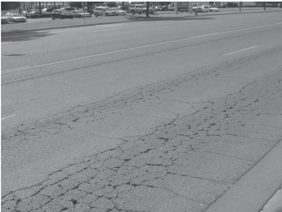
FIGURE 1.17 Fatigue failure of asphalt pavement due to repeated traffic loading.
