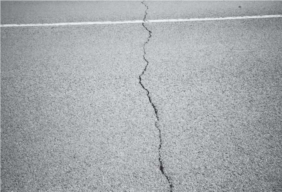
FIGURE 9.12 Thermal cracking resulting from the use of too-stiff asphalt in a cold climate area. (Courtesy of FHWA)
