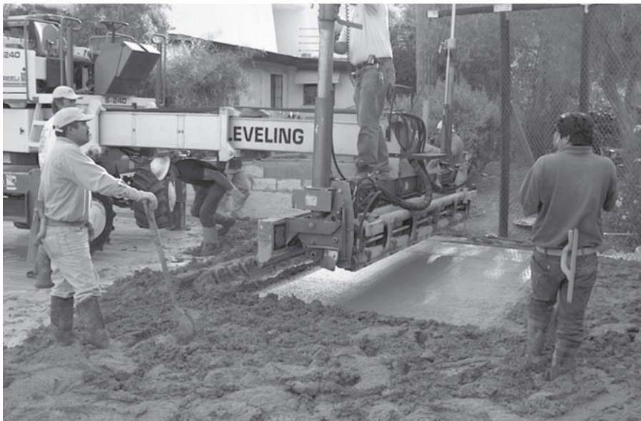
FIGURE 7.23 Using laser level to establish elevation for finishing concrete. (Courtesy of FHWA)
