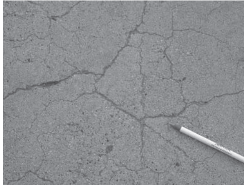
FIGURE 5.19 Example of cracking in concrete due to alkali-silica reactivity.
