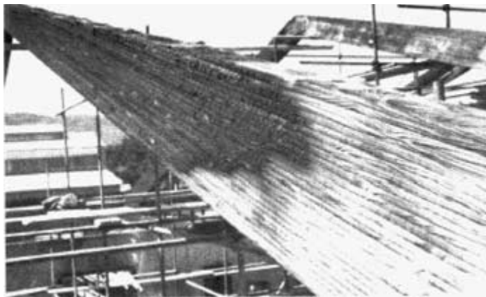
FIGURE 6.21 Wood fire damage 2. (From Ref. 13, p. 275. With permission, John Wiley & Sons, Limited, from Buchanan, Andrew H., Structural Design for Fire Safety , Copyright 2001.)
