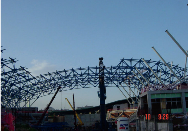
Fig. 8.23. Erection of the central part of a large opening structure follows erection of the end parts
