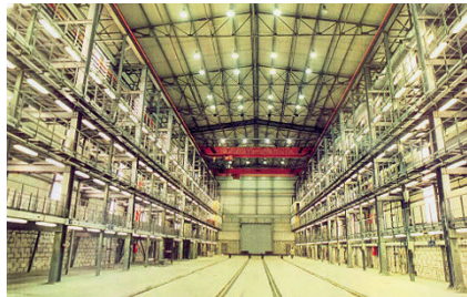
Fig. 6.28. Shipyard building having built-up columns with batten plates up to the level of the runway beams
