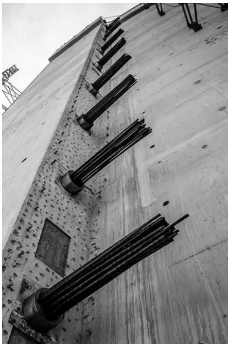
Figure 3.13 Prestressing anchorages at a buttress of a prestressed tank. (Courtesy of VSL International Limited, Hong Kong, China.)
