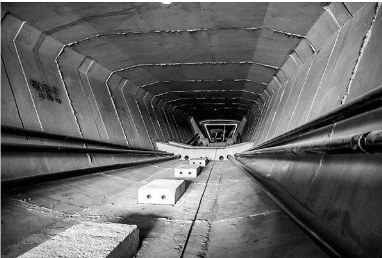
Figure 3.14 External tendons in bridge box girder section. (Courtesy of VSL International Limited, Hong Kong, China.)
