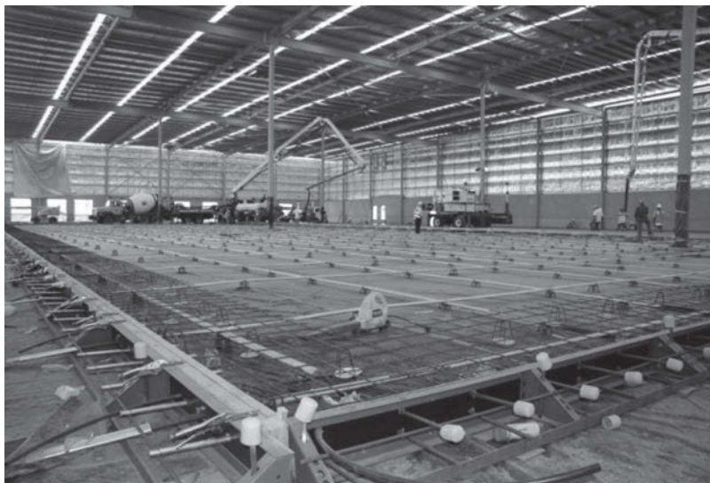
Figure 3.3 Examples of post-tensioned slabs before concrete casting. (Courtesy of VSL Australia Limited, Sydney, New South Wales, Australia.)
