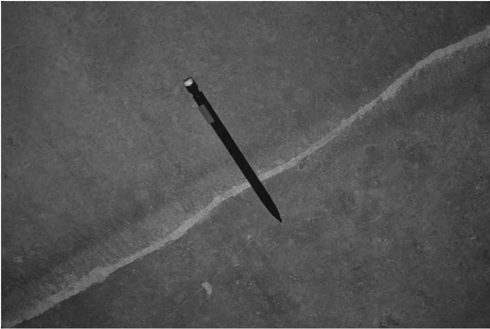
Figure 13.4 This crack was patched with semi-rigid epoxy. Not every crack patch looks this good, however
