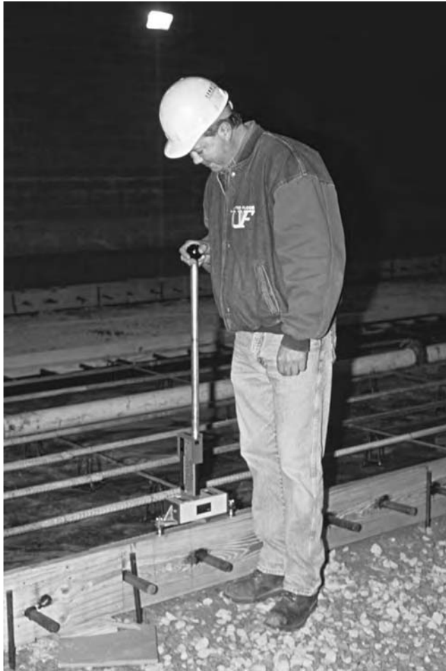
Figure 11.11 Using an electronic level to check a timber form on a superflat job
