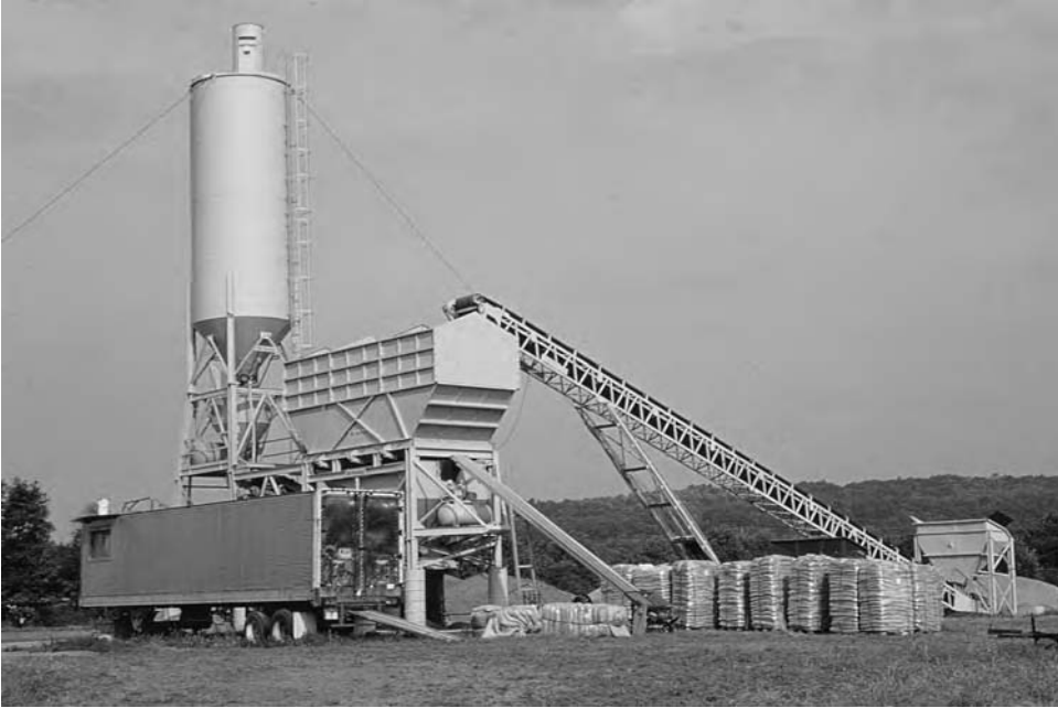
Figure 10.1 Temporary batch plant near the job site
