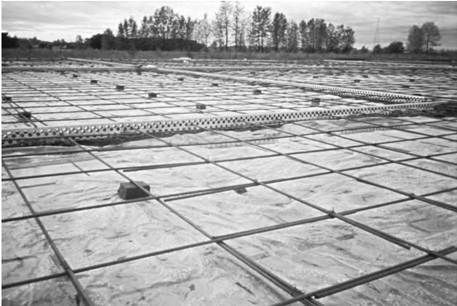
Figure 16.3 Light reinforcement for crack control in a jointed slab – 12-mm (#4) bars spaced 600 mm (24 in) on centre
