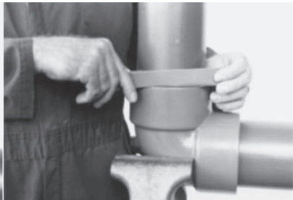
Remove excess cement residue at pipe joint and make sure the joining is moisture-free.
