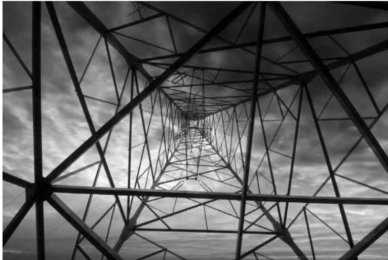
FIGURE 11–1 (See color insert.) Trusses are rigid networks of simple two-force members and provide the framework for many structures such as this tall tower. Each member of this tower is long relative to its cross section, so any that is loaded in compression is susceptible to buckling. Care must be taken to ensure that no single member of this structure buckles resulting in a sudden and catastrophic failure of the entire structure.
