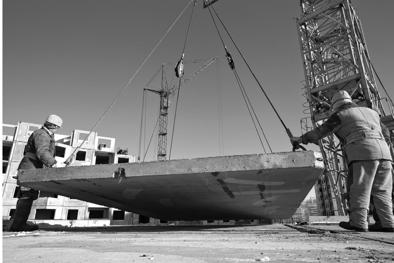
FIGURE 1-1 (See color insert.) The concepts of strength of materials are critical in many applications, including this one where workers assure that this concrete element is ready to be lifted into place where it will serve as a critical piece of a multistory structure.
