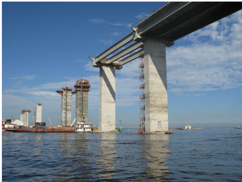
FIGURE 5-1 A bridge under construction shows vertical supports in place where beam reactions will occur. One can see that the effect on each beam in the completed bridge will vary with respect to position relative to those supports. In this chapter, we will learn to quantify what is happening internally along the length of a loaded beam so that, in a subsequent chapter, we will be able to calculate stress and deflection in beams.
