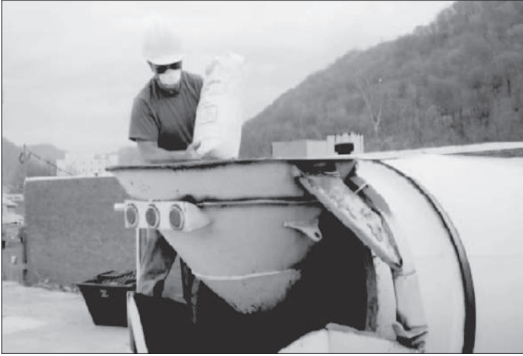
Adding repulpable bags of densified silica fume directly to truck mixer for precautions regarding unopened bags. Note the use of a dust mask and safety glasses.
