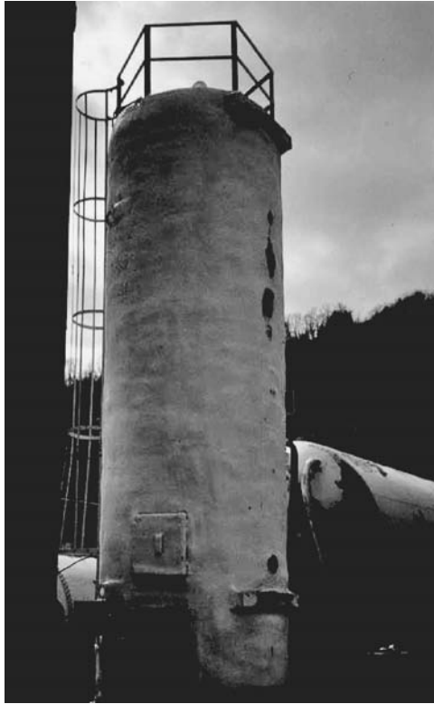
FIGURE 6.12 Silica fume storage in silos.
