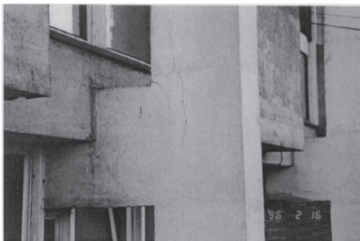
Figure 6.1 Structural cracks at a column beam connection.
