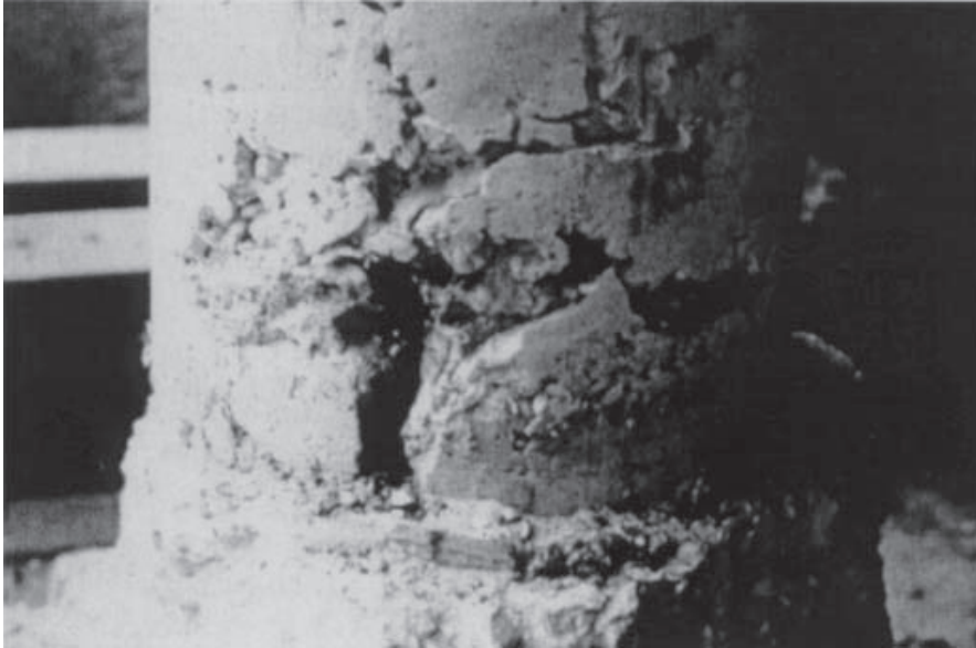
Figure 6.8 Poor quality construction.
