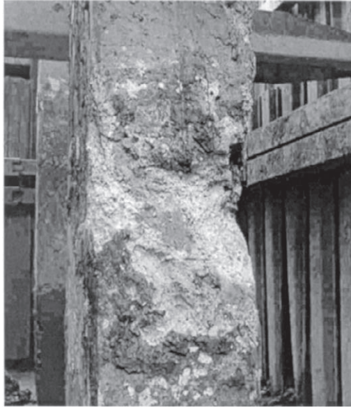
Figure 6.5 Foundation damaged by thaumasite attack.
