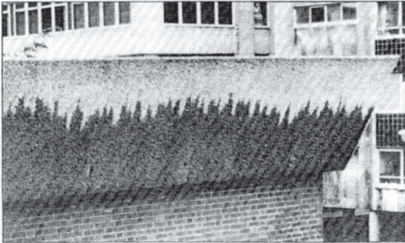
Figure 19.16 Partial washing caused by water running off a horizontal surface.
