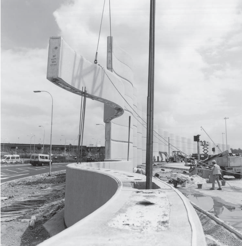
Figure 21.7 Gatwick Airport: Acoustic wall. Erection in progress, preparing to thread an element onto continuity steel, the operation to be completed by grouting after positioning the eighth tier element. (Courtesy Gatwick Airport Ltd ( BAA plc), The Pavement Team (AMECJV) and C.V. Buchan.)
