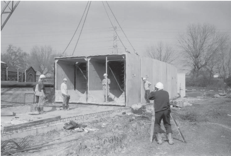
Figure 21.8 Setting one of a batch of precast culvert elements onto a prepared foundation. Note the absence of falsework and formwork. ( Courtesy Hanson Concrete Products Ltd. )
