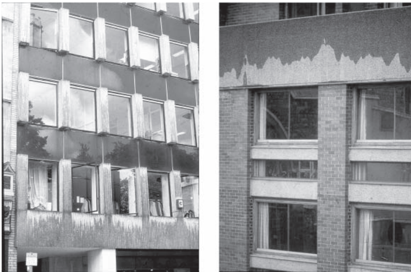
Figure 19.6 Concrete appears much darker when it is wet.
