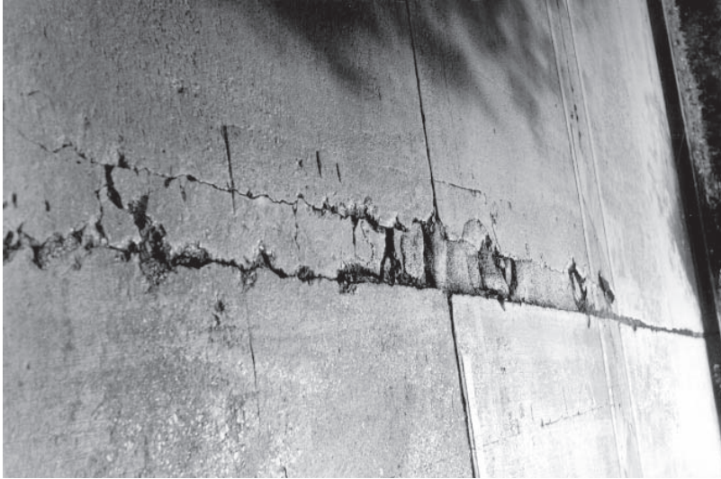
Figure 22.18 Badly bonded tie bars.
