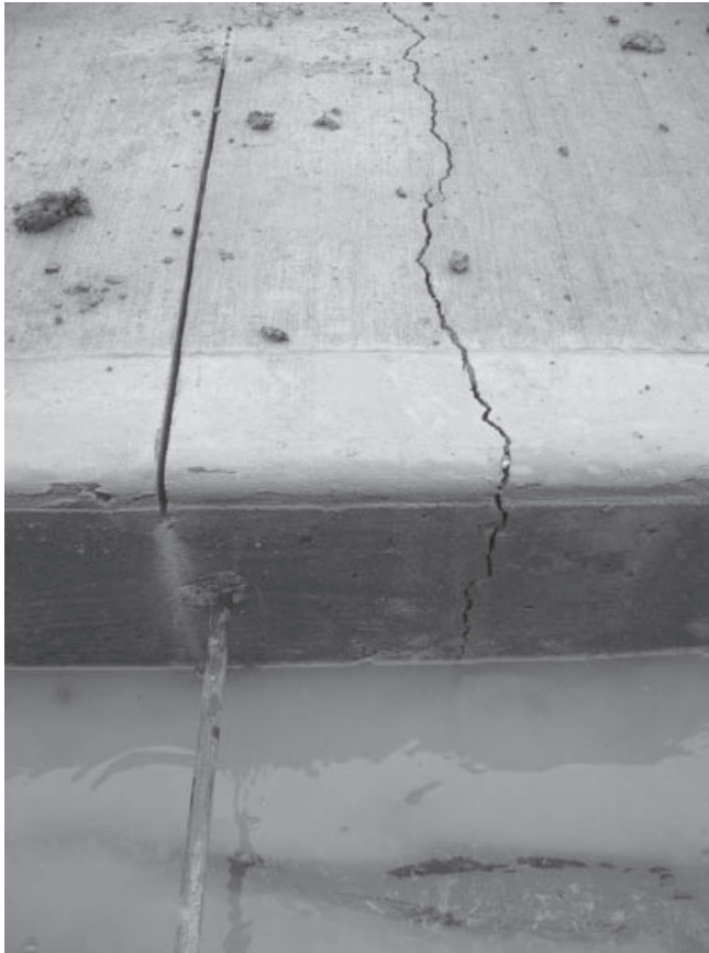
Figure 22.15 Joint cut too shallow.
