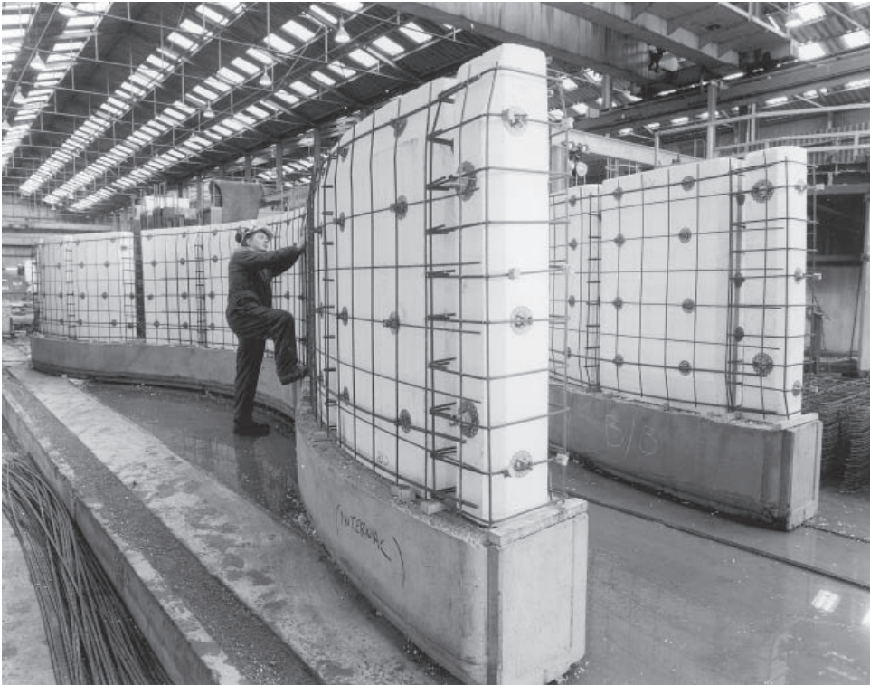
Figure 21.5 Gatwick Airport: Acoustic wall. Setting up the core formers and reinforcement for the waveform wall. Architectural quality concrete, counter-cast to ensure fit. (Courtesy Gatwick Airport Ltd (BAA plc), the Pavement Team (AMECJV) and C.V. Buchan.)
