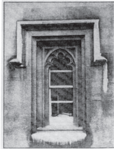
Figure 19.5 An even layer of dirt on a north-facing stone wall being affected by concentrated flows of water.
