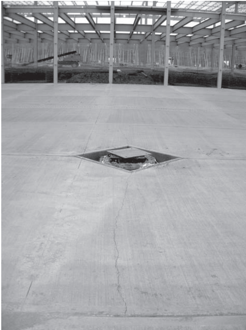
Figure 22.14 Joint cut too late and incorrect joint location.
