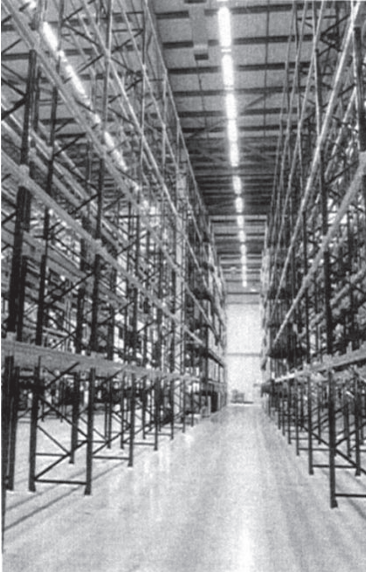
Figure 24.9 Typical pallet racking system – wide aisle (Note: no bottom beam in this system).
