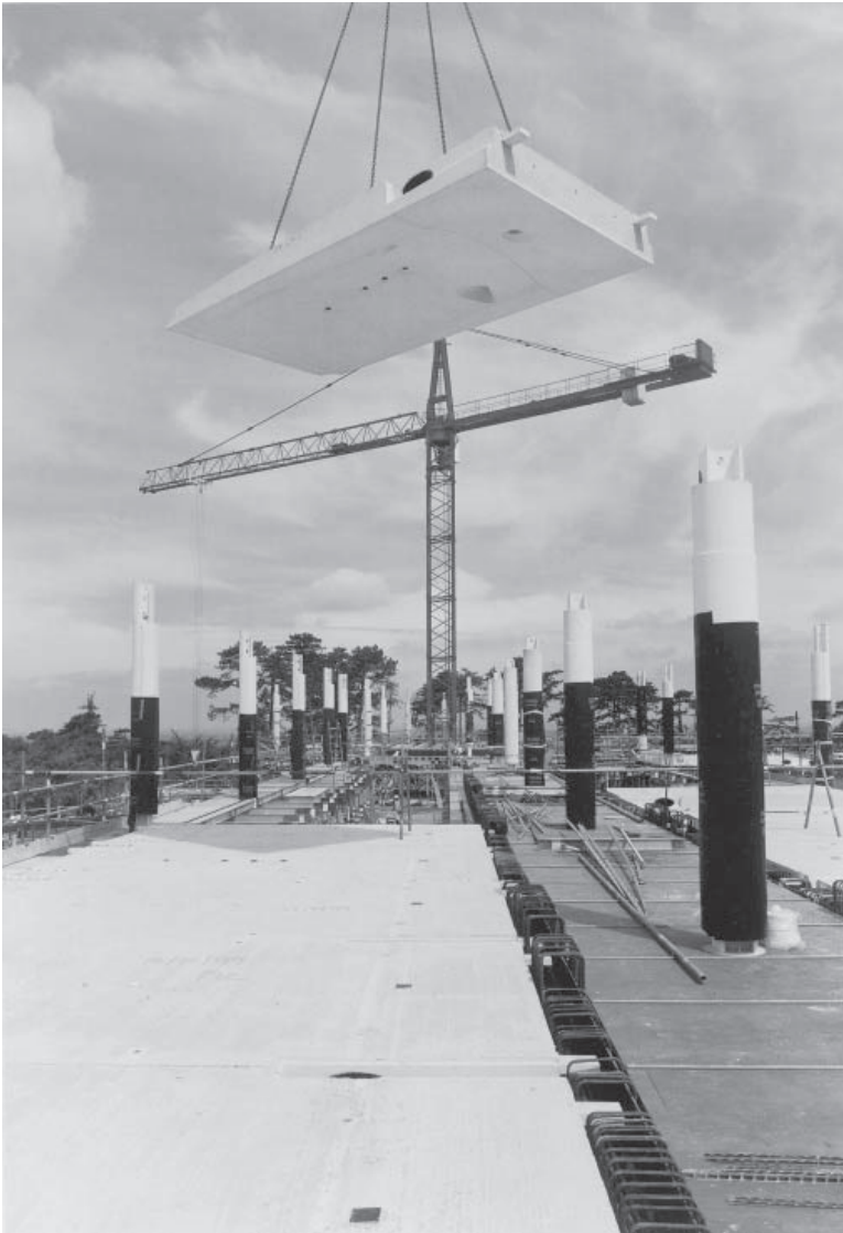
Figure 21.4 Toyota (GB) Ltd, Head Office: Precast concrete two-storey columns and self-finished floor elements combine with in-situ concrete beams and floor topping to enhance the buildability of a cost-effective structure. (Courtesy Takaneke (UK) Ltd and Trent Concrete Ltd.)
