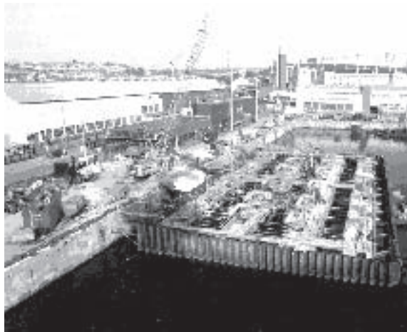
Figure 13.18 LLRF facility at Devonport.
