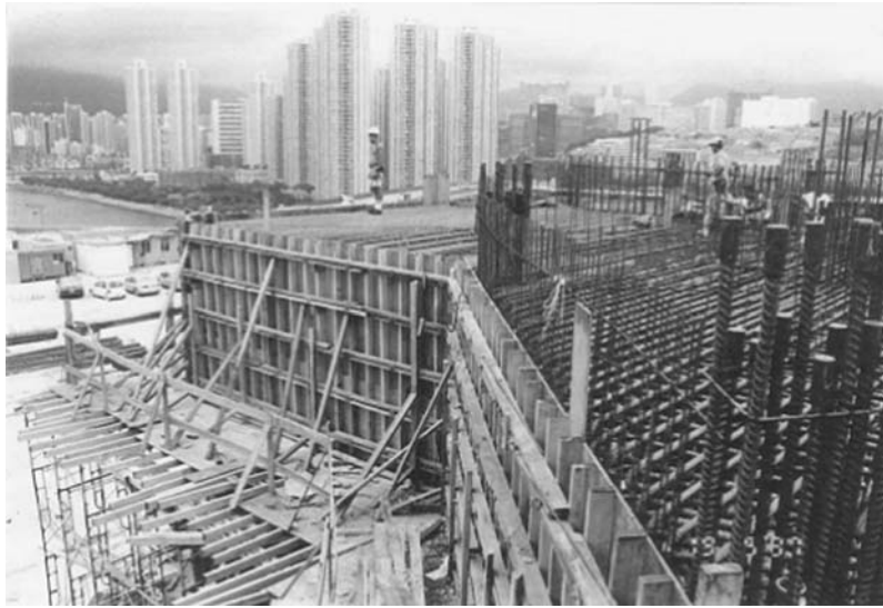
Figure 3-15 Framework for transfer block of a tall building (photo provided by Peter Allen)
