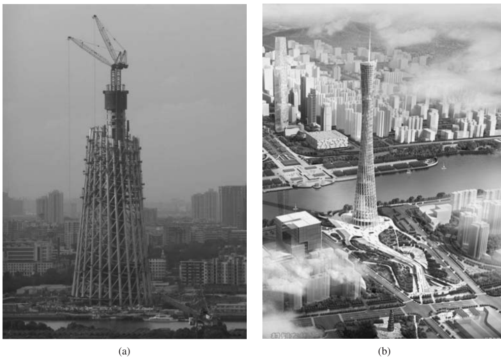
Figure 6-54 (a) Guangzhou TV Tower under construction and (b) site view of finished tower in China (Photo provided by Linhai Han)
