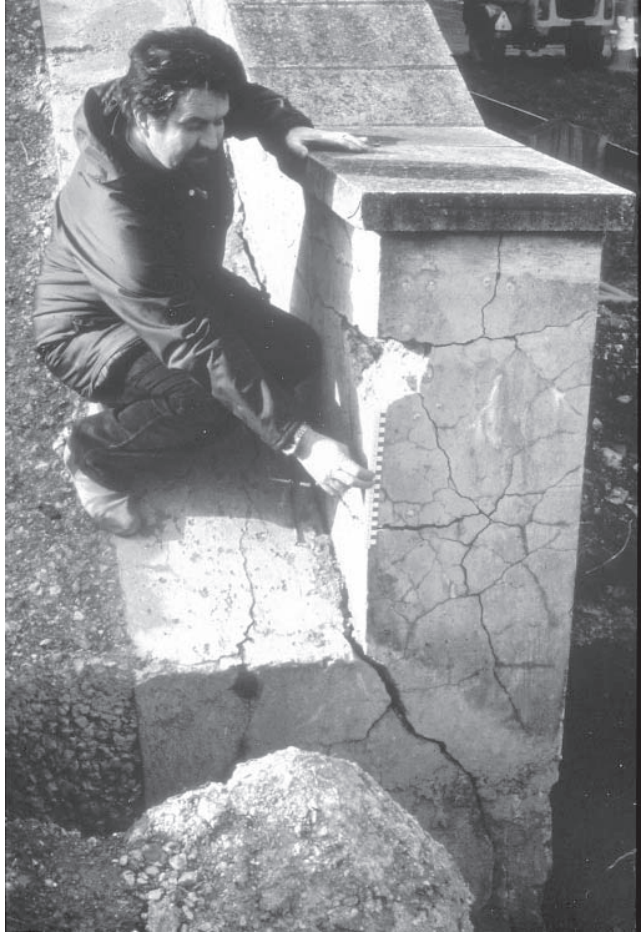
Figure 13.1 ASR cracking and displacement in a highway bridge wing wall, UK.
