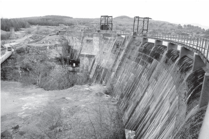
Figure 13.14 Maentwrog Dam in Wales: a case of ASR damage caused by greywacke aggregate.
