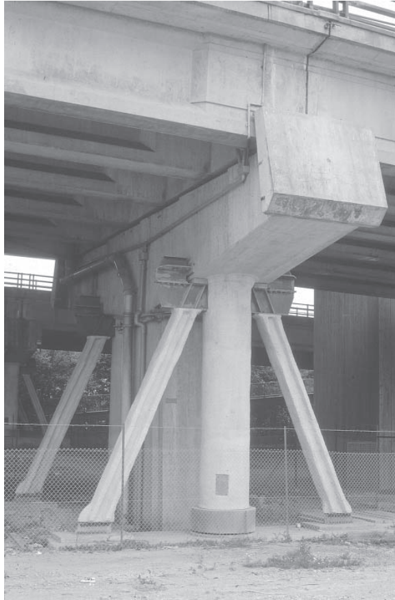
Figure 13.20 Auxiliary support for pier and pile cap affected by ASR: Marsh Mills Viaduct, Plymouth.
