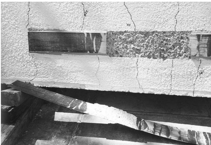
5.4 Close-up showing splitting within the prefabricated strip.
