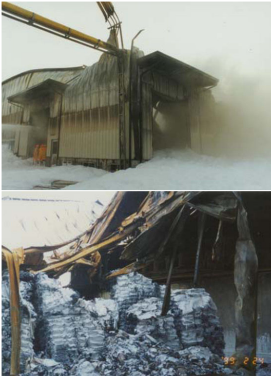
Fig. 11.2 Damage to steel portal frames caused by a fire
