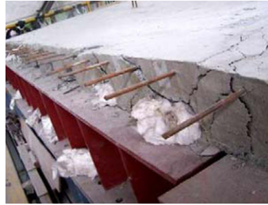
Fig. 9.20 Cracks along the short side edge on S-1
