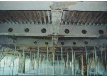
(c) Large deflection in the steel beam
