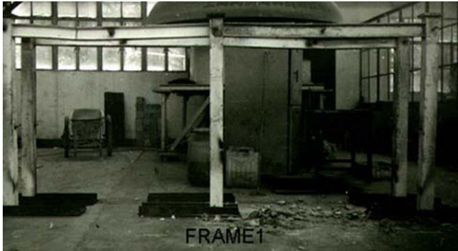
(a) Failure of FRAME 1
