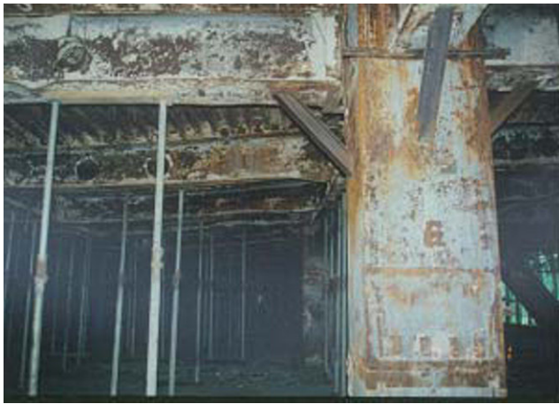
Fig. 7.18 Damage to the beam-column connection by a fire
