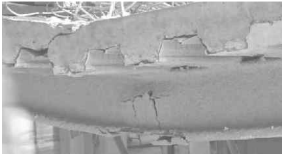
Fig. 5.11 Failure of the composite beam
