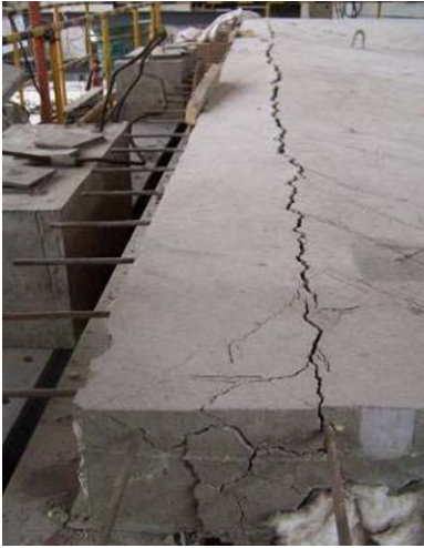
Fig. 9.19 Cracks along the long edge on S-1
