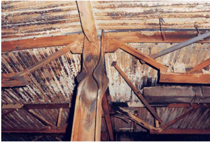
Fig. 1.2 Buckling of the column in a fire
