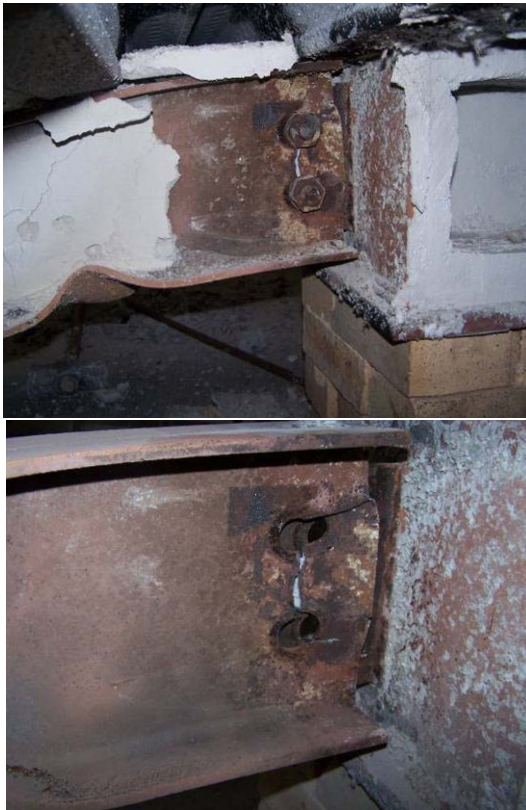
Fig. 7.40 Breaking of the joint in test CB150
