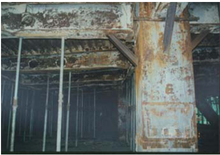
(a) Fracture of the beam-to-column connection
