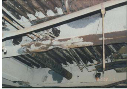
(b) Local buckling of the steel beam
