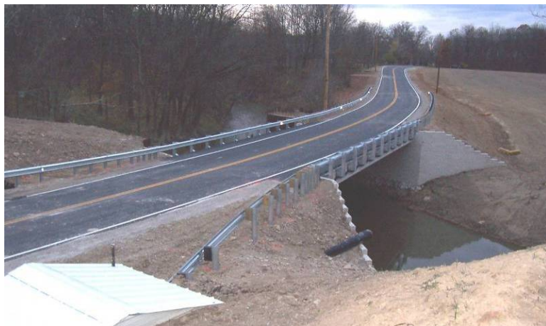
Figure 5.3.2.4-1 GRS-IBS Bridge Example Top Photo: GRS Abutment During Construction Bottom Photo: Completed Bridge (built in 47 days) (source: Defiance County Ohio)
