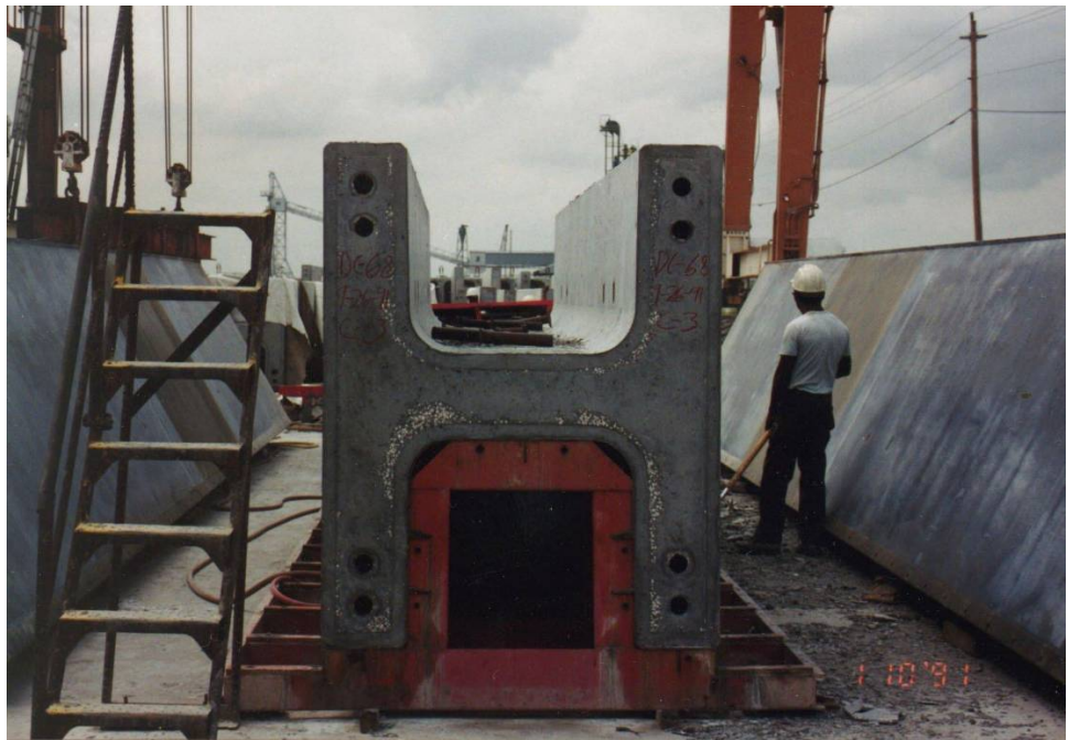
Figure 5.3.1.1-1 Precast Open Frame Pier Bent Top Photo: Overall Bridge Bottom Photo: Casting of Columns (source: Splice Sleeve North America Inc.)
