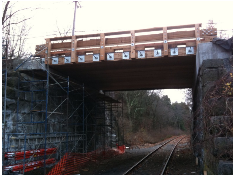
Figure 5.2.4.3-1 Stress Laminated Timber Deck Span Top Photo: Panel Erection Bottom Photo: Final Post-tensioning (source: Massachusetts DOT)
