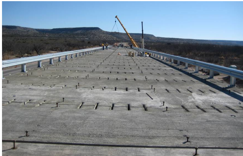
Figure 2.6.1.1-4 Precast Deck Panel Project in Texas Based on NCHRP Report 584 Details (source: Texas DOT)
