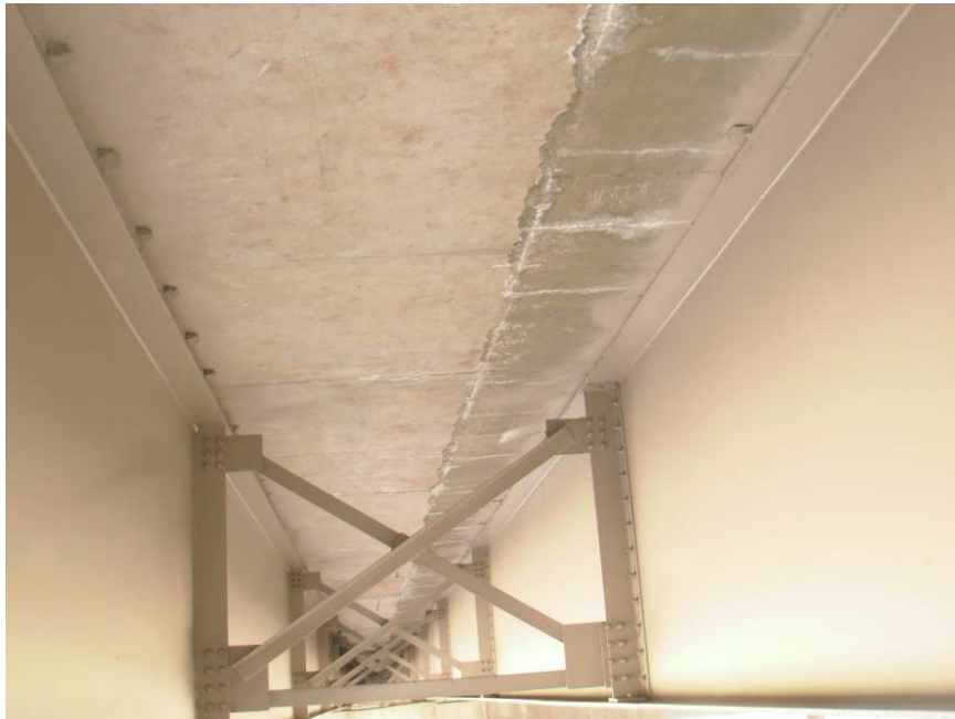
Figure 7.8-1 Cracking in Closure Pour Concrete
