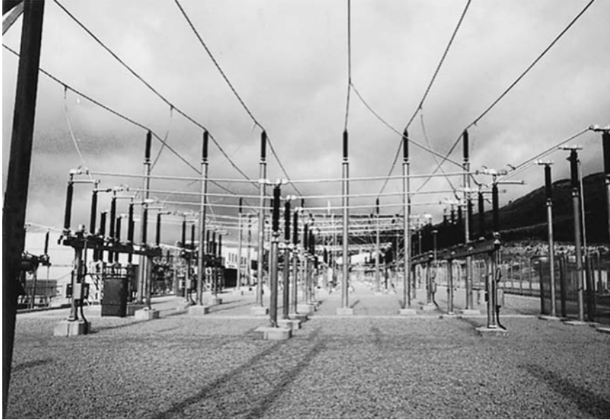
Figure 18.16 'Tarantula' 132 kV busbar
