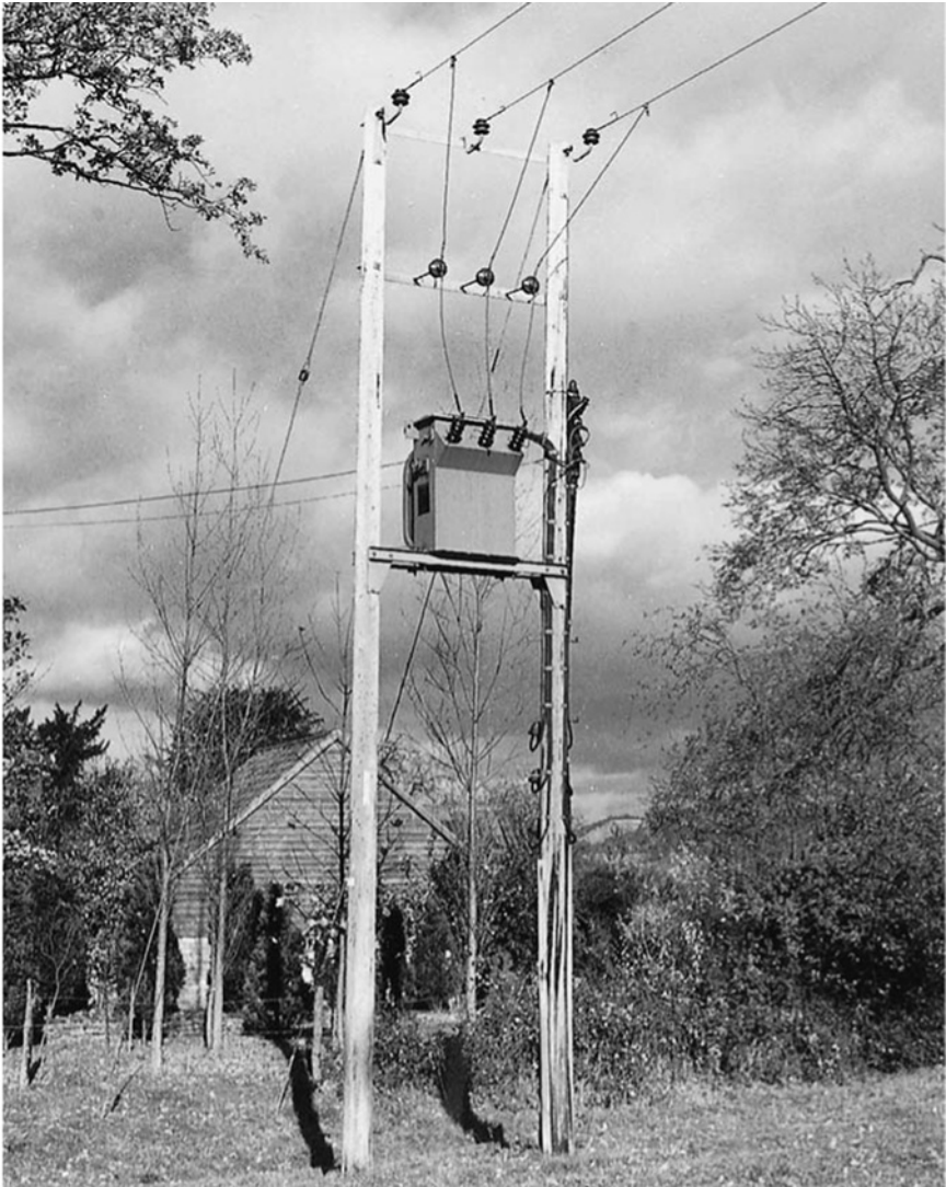
Figure 17.13 Pole-mounted 11/0.415 kV transformer and LV distribution
