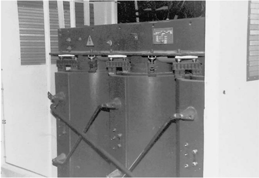
Figure 14.24 1 MVA, 21/0.4 kV, cast resin transformer
