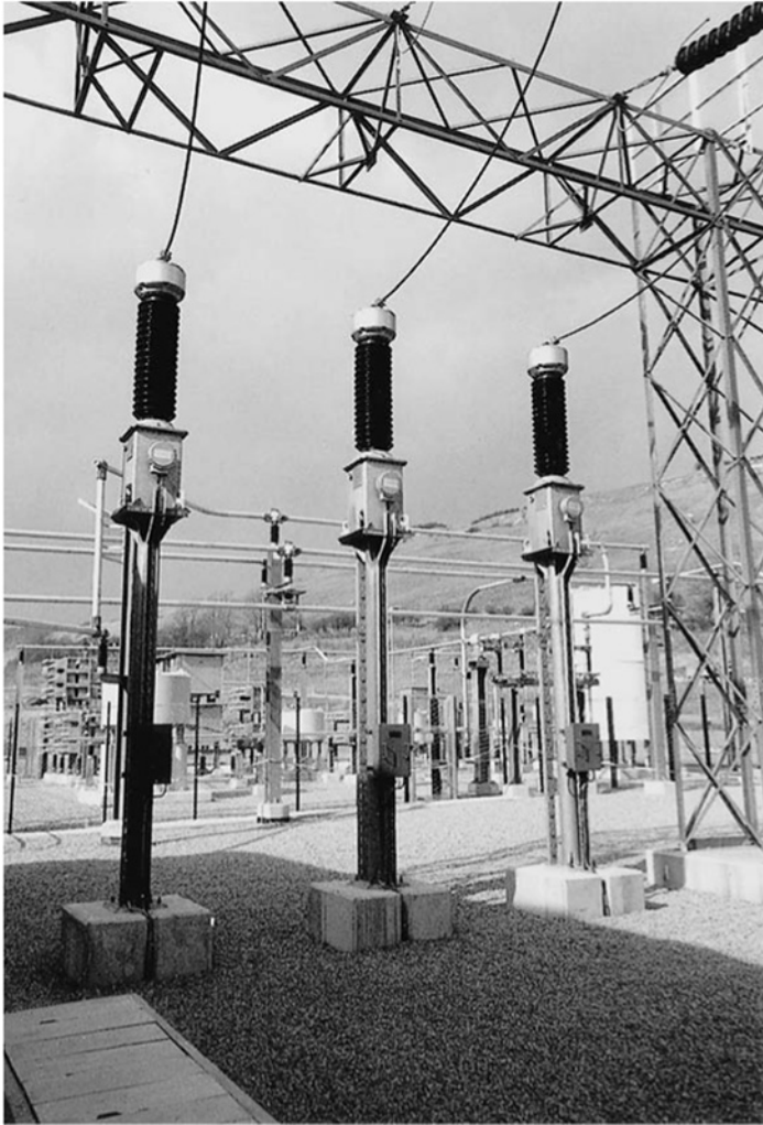
Figure 17.5(b) 132 kV gantry bolted connected – Channel Tunnel, Folkestone
