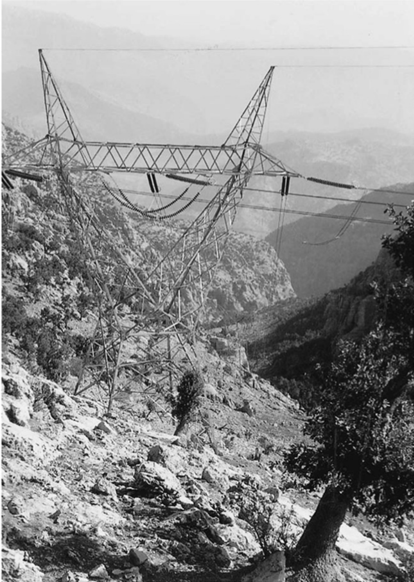
Figure 16.2 400 kV single circuit twin conductor overhead line crossing the Zagros Mountains in Iran (courtesy of Balfour Beatty)
