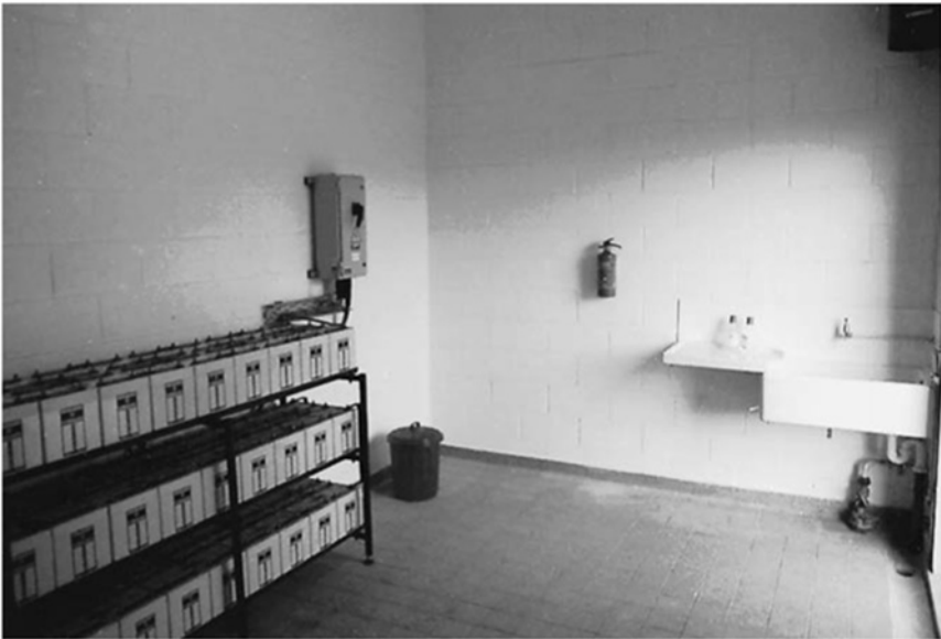
Figure 4.3 Primary substation battery room DC distribution and charger (courtesy of Balfour Beatty Projects and Engineering Ltd)
