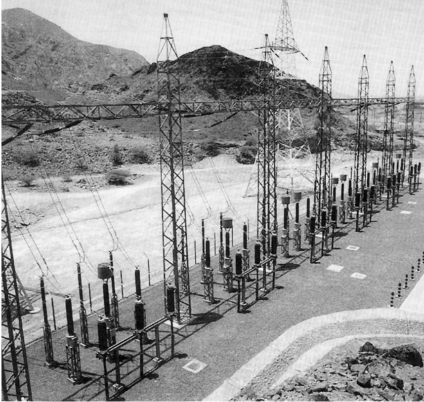
Figure 21.11(b) Qaboos 132 kV substation, Oman-OHL incomers with surge arresters, CVTs/line traps and cable sealing ends
