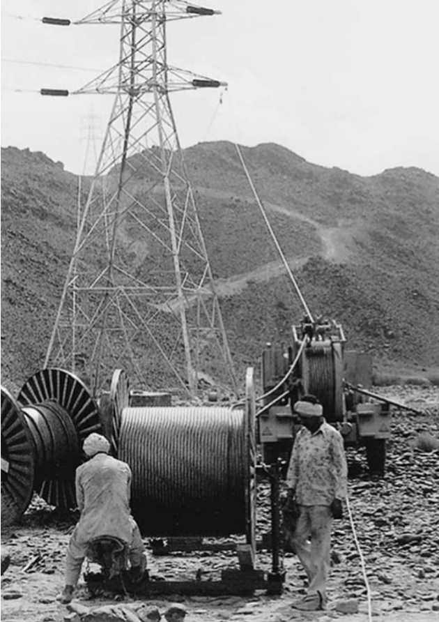
Figure 18.21 Conductor running out in progress. Tensioner and drums at 60 degrees angle tower. United Arab Emirates – 132 kV East Coast Transmission
