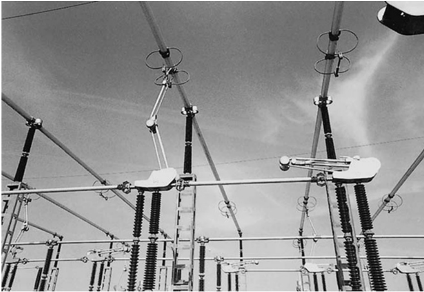
Figure 13.9(d) Pantograph disconnector
