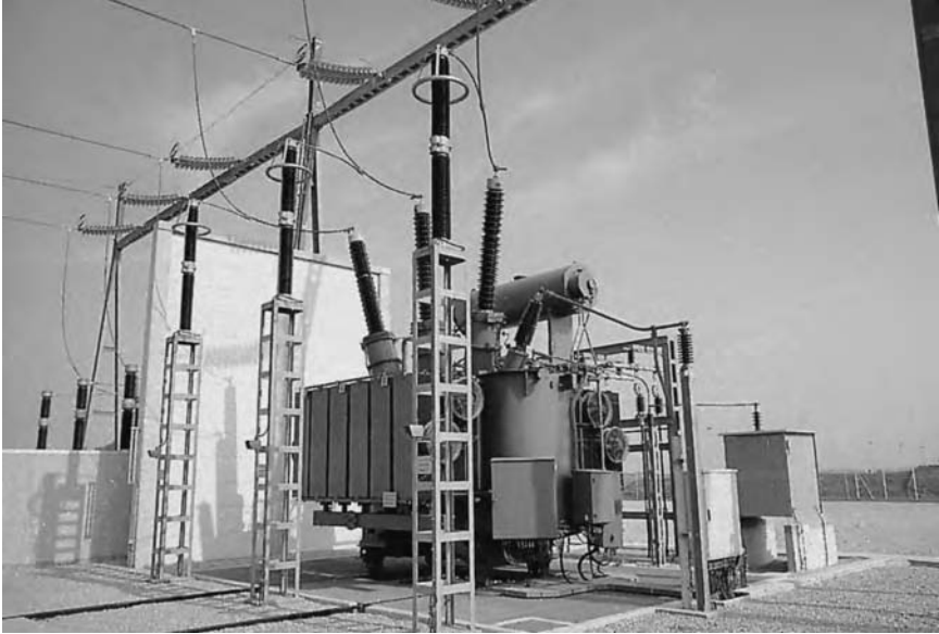
Figure 14.22 225/21 kV, 35/40 MVA, ONAN/ONAF transformer at Coquelles substation, France
