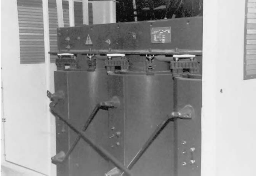
Figure 14.24 1 MVA, 21/0.4 kV, cast resin transformer
