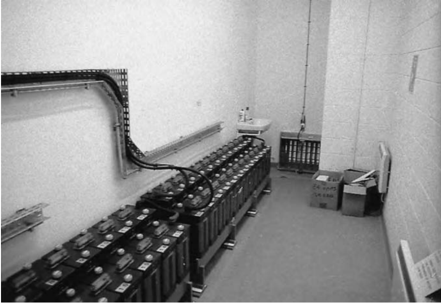
Figure 4.11 Conventional vented lead acid battery room showing battery bank, sink, tiles and ventilation arrangements
