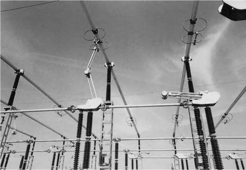
Figure 13.9(d) Pantograph disconnector
