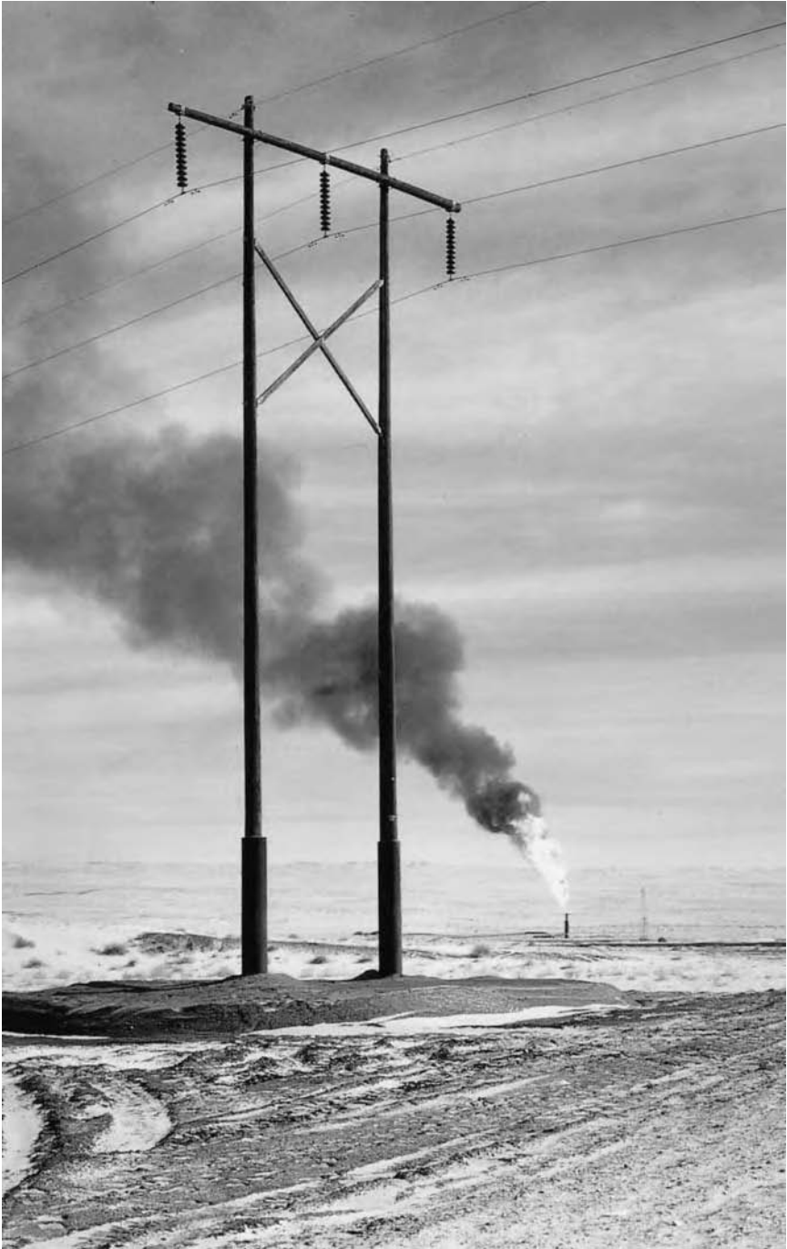
Figure 17.12 115kV twin pole, single circuit line – Saudi Arabia
