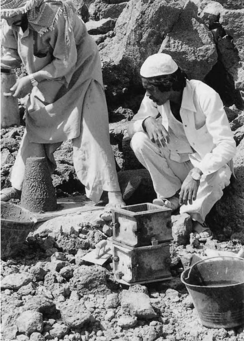
Figure 15.8 Concrete cube and slump cone samples being prepared – Yanbu-Medina 380 kV transmission line, Saudi Arabia (courtesy of Balfour Beatty Projects and Engineering)
