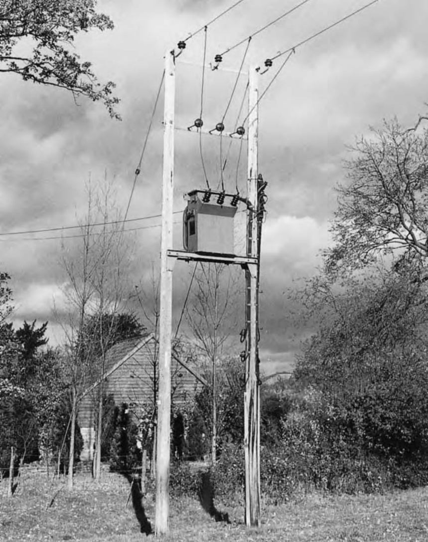
Figure 17.13 Pole-mounted 11/0.415 kV transformer and LV distribution
