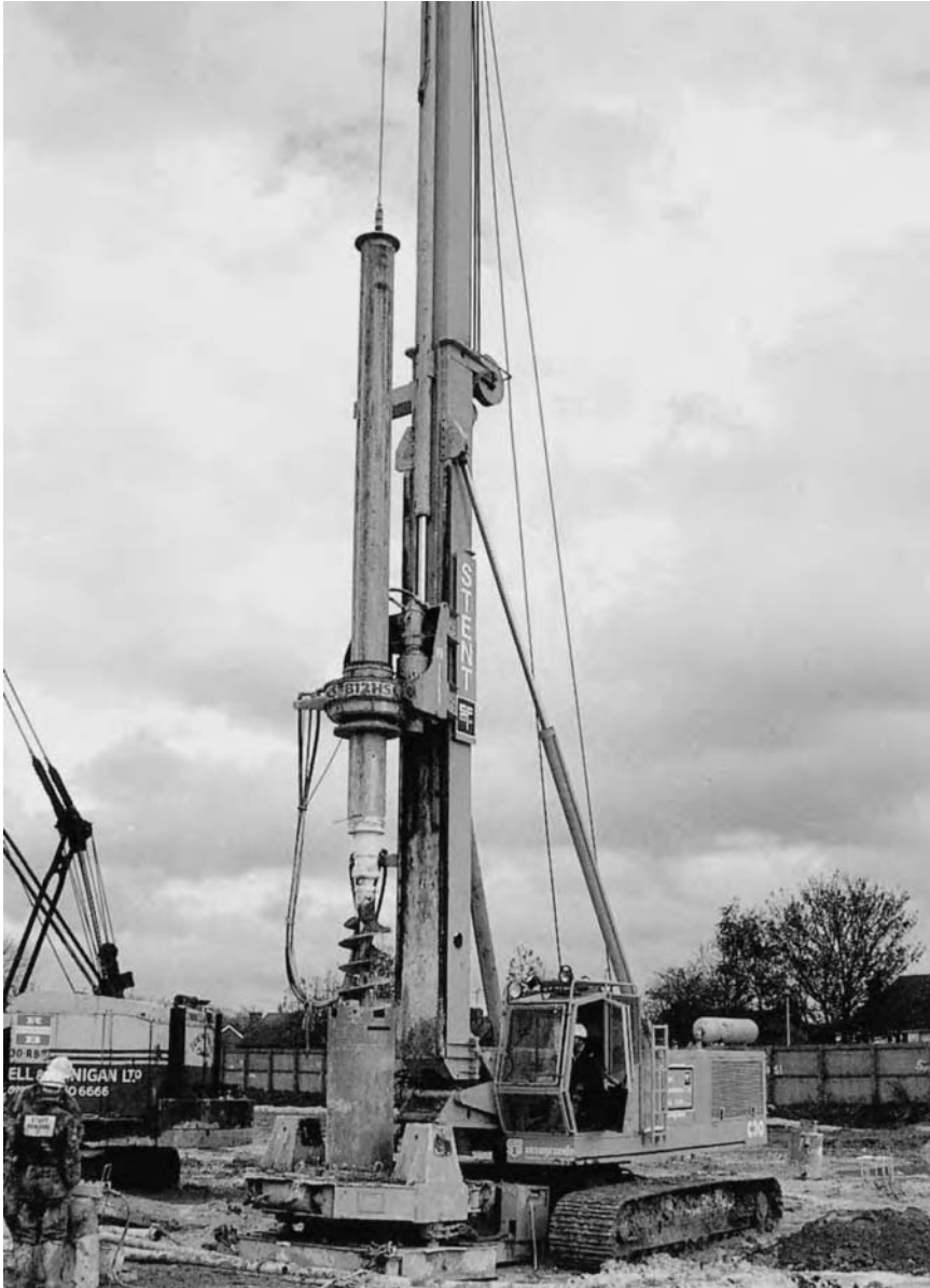
Figure 15.5 (b) Auger for forming cast in-situ concrete piles – 400 kV Sellindge substation, Kent
