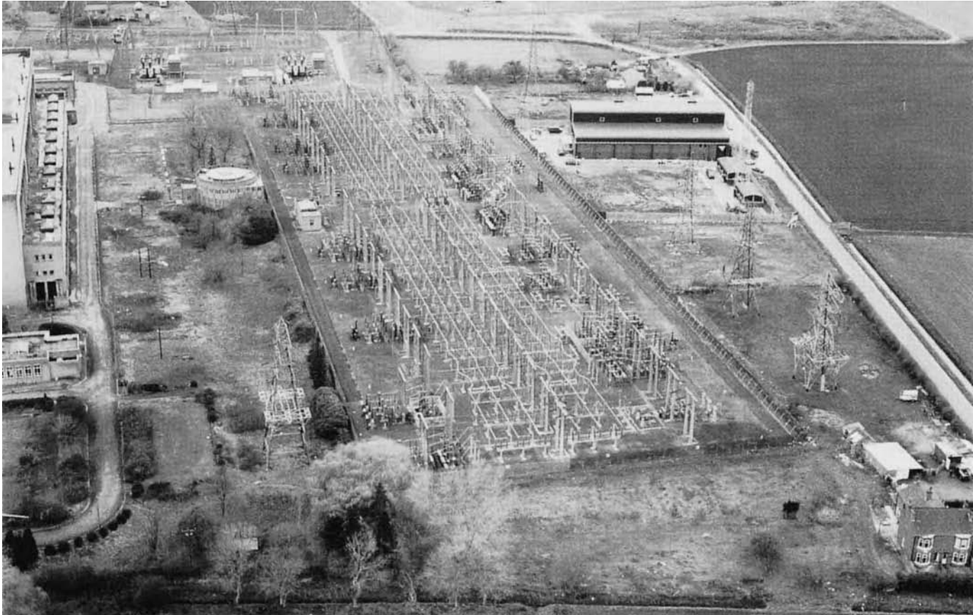
Figure 3.1 GIS substation replacement for conventional open terminal outdoor arrangement. A striking comparison between land area requirements for a conventional open terminal 132 kV double busbar switchyard arrangement and replacement indoor GIS housing to the top right-hand corner of the picture (Yorkshire Electricity Group plc)
