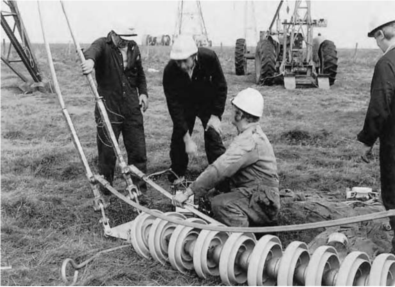
Figure 17.15 400 kV cap and pin insulator set. Low resistance 'ducter' testing on connections in progress
