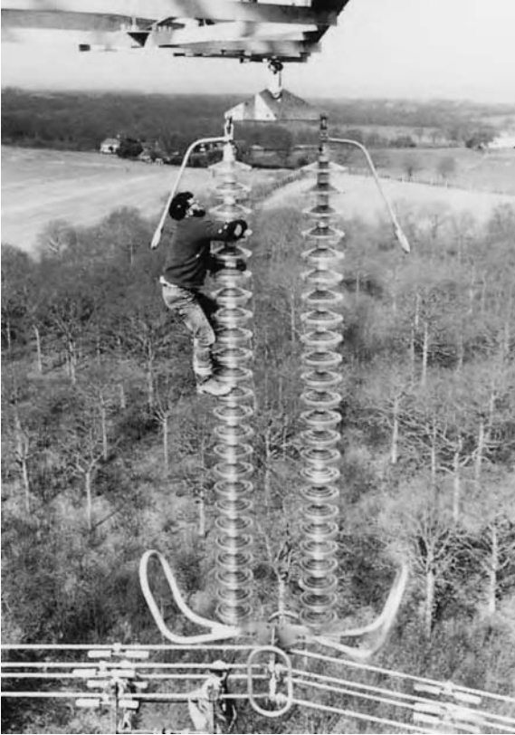
Figure 18.18 400 kV Lydd-Bolney (UK) overhead line—quad conductor glass insulators showing arcing horns and stockbridge dampers
