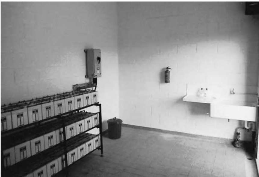
Figure 4.3 Primary substation battery room DC distribution and charger (courtesy Balfour Beatty Projects and Engineering Ltd)
