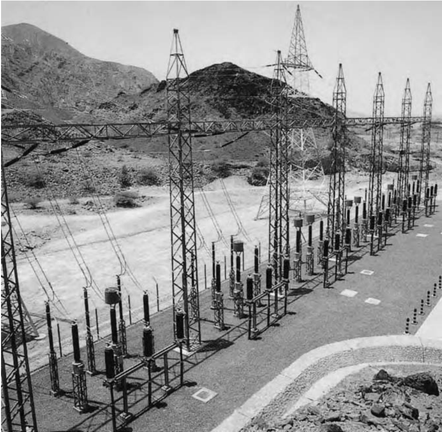
Figure 21.11(b) Qaboos 132 kV substation, Oman—OHL incomers with surge arresters, CVTs/line traps and cable sealing ends
