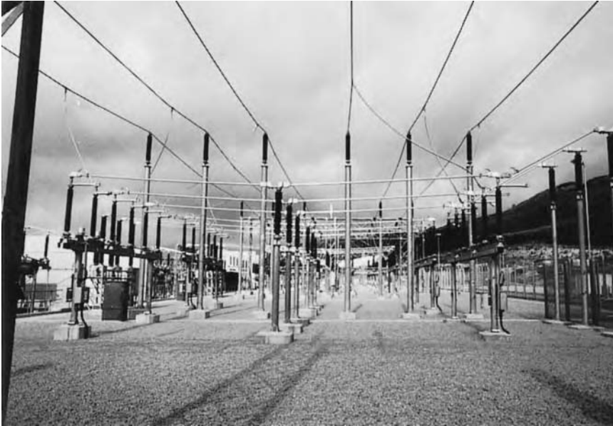
Figure 18.16 'Tarantula' 132kV busbar
