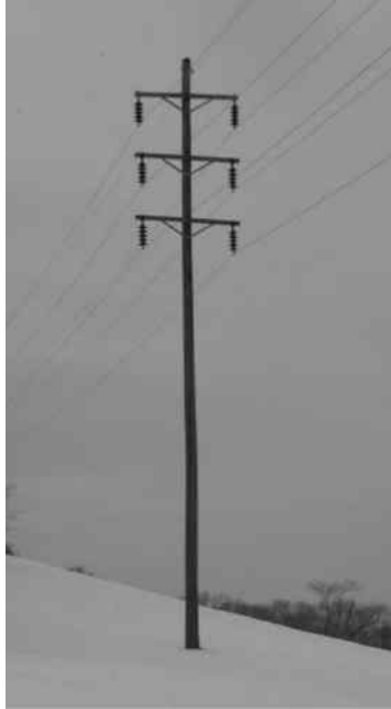
FIGURE 2.6 Medium-voltage distribution tower. (Photograph by author.)
