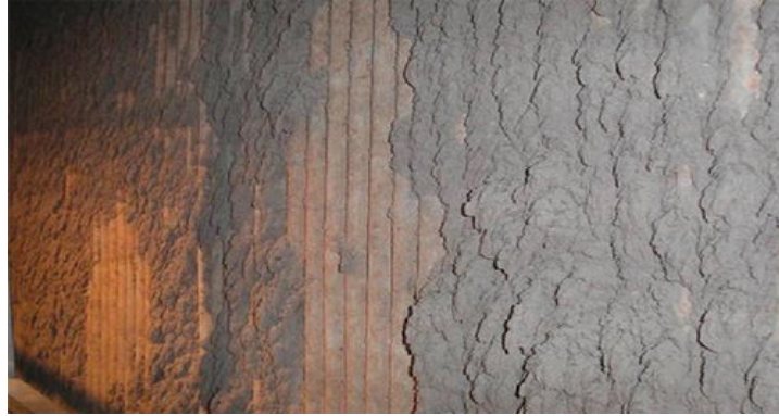
FIGURE 5.2 Slagging accumulation on the water wall surface of a boiler furnace.
