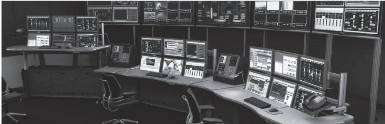
Figure 8.3 (b) Typical control room showing operator displays. © Emerson, reproduced with permission
