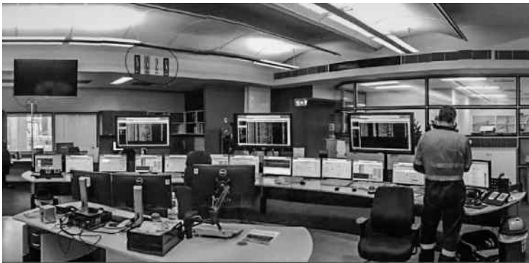
Figure 12.3 New control room for the four-unit gas-fired plant. Control consoles for four other units of an adjacent station were also located in the same room. Note the 'Yarway' drum level indicators (circled). © AGL Energy Ltd. Used with permission
