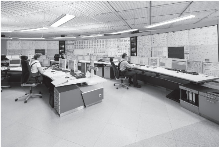
Figure 8.3 (a) Typical control room. © ABB, reproduced with permission
