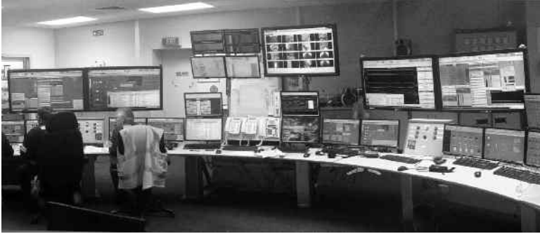
Figure 12.5 Replacement HMI for both units and common (station) plant, located in a different area of the same control room. © Millmerran Operating Company. Used with permission
