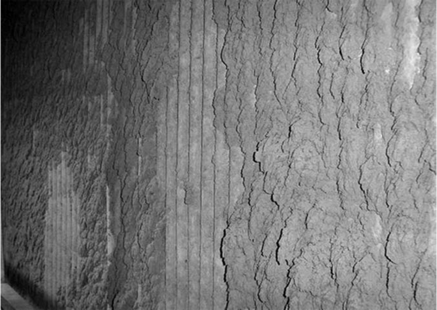
Figure 24: Example of fouled water tube furnace wall [23].
