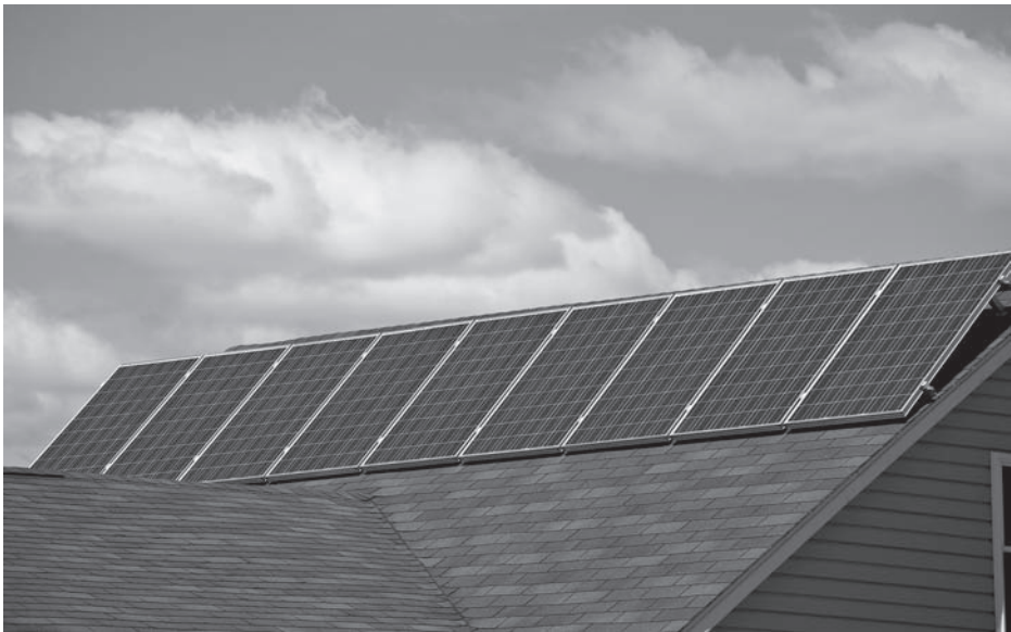
FIGURE 14-3 A roof-mounted solar array is unobtrusive.
