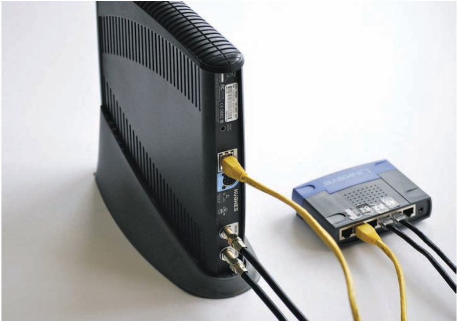
FIGURE 11-6 Modem for Internet access satellite dish system. Notice the two coaxial cables, one for receiving and one for transmitting, that come from the dish. A Category 5e cable feeds the modem output to an Ethernet hub, which is necessary because two computers are connected.
