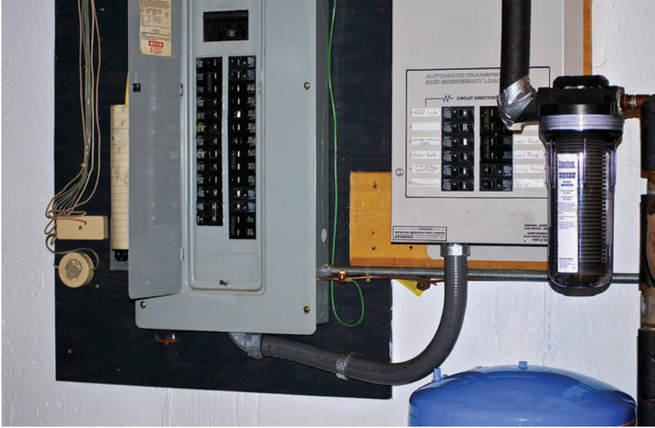
FIGURE 5-4 Note the clear violation of working-space requirements.
