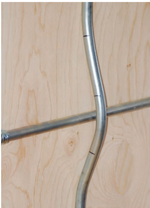
FIGURE 7-13 A three-point saddle bend, which is used where a single pipe must be crossed.
