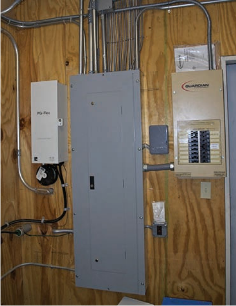
FIGURE G-20 A limited number of selected circuits are chosen to be energized by the alternate power source during a utility outage.
