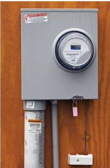
FIGURE G-11 The intersystem bonding termination, in the small white plastic enclosure below the meter socket, is a required part of every new service.
