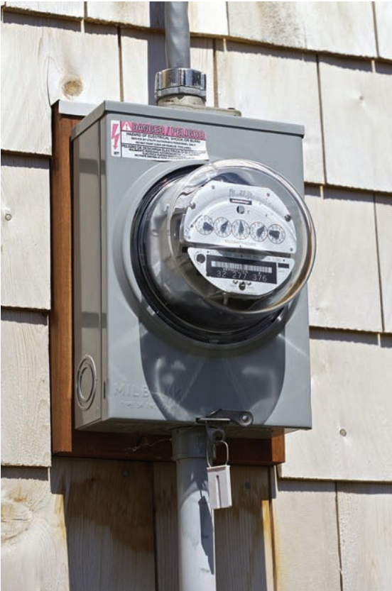
FIGURE 4-5 This meter socket is in back-to-back configuration with the entrance panel on the inside of the house. The polyvinyl chloride (PVC) conduit coming out of the bottom of the meter socket contains the grounding-electrode conductor.
