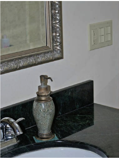
FIGURE G-19 Rocker switches combined with a ground-fault circuit interrupter (GFCI) are an attractive feature in this upscale bathroom.
