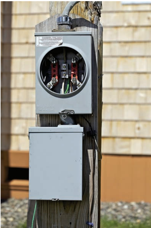
FIGURE 4-3 A temporary service. The two GFCI circuits need to be connected, and then it will be time to call the utility.
