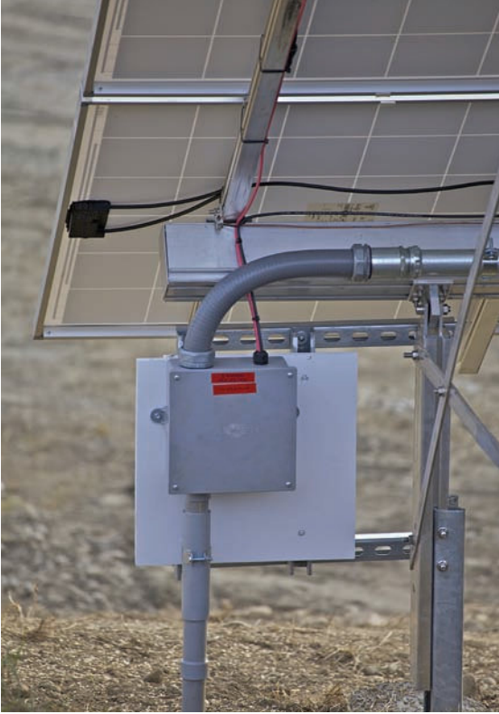
FIGURE 7-3 Underground raceway placement must be coordinated with equipment position if the conduit riser is to be plumb.
