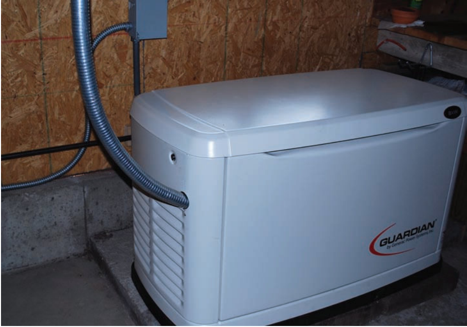
FIGURE 13-1 A small high-end generator.
