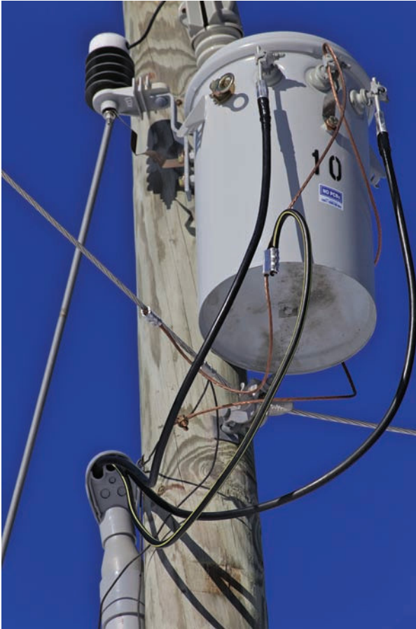
FIGURE G-21 A pole-mounted transformer connected to the service for an individual home.
