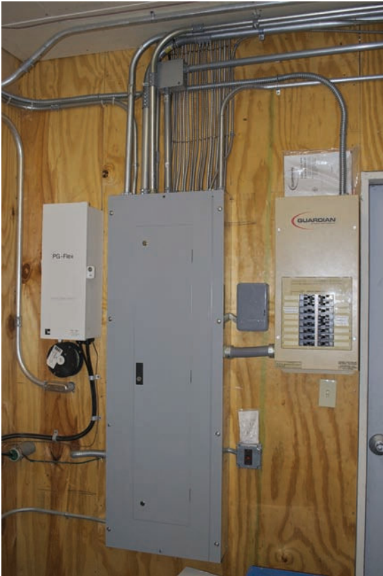
FIGURE 13-3 The automatic transfer switch often performs other functions, such as sensing a utility outage, starting the generator, and returning to utility power after the outage has ended.
