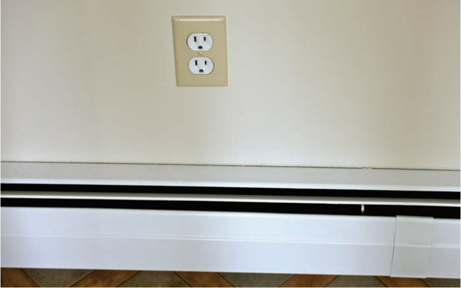
FIGURE G-16 This wall receptacle is improperly located above a baseboard heat unit.
