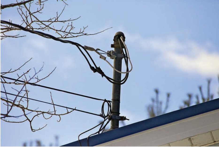
FIGURE 4-1 For this aerial masthead service, the point of connection consists of the crimped splices upstream from the weather head. (The cable TV and telephone cables attached to the service mast are a Code violation.)
