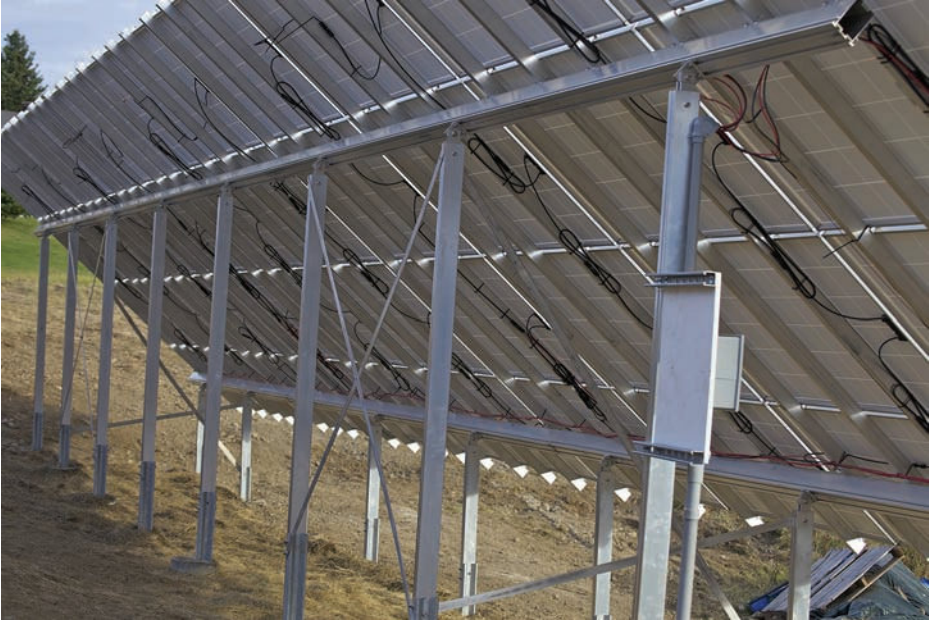
FIGURE 14-5 Sonotube concrete footings should not be too far out of the ground so as to limit pitting from the weather.
