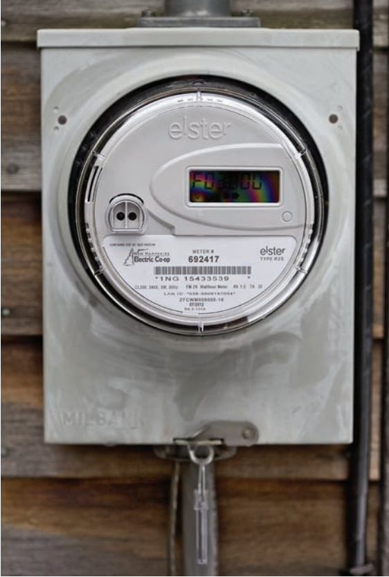
FIGURE 15-1 This smart meter has a two-way wireless connection to the utility.
