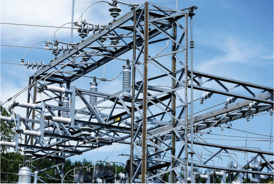
FIGURE 15-2 The substation is the source of local power, and the utility controls all lines that emanate from it.
