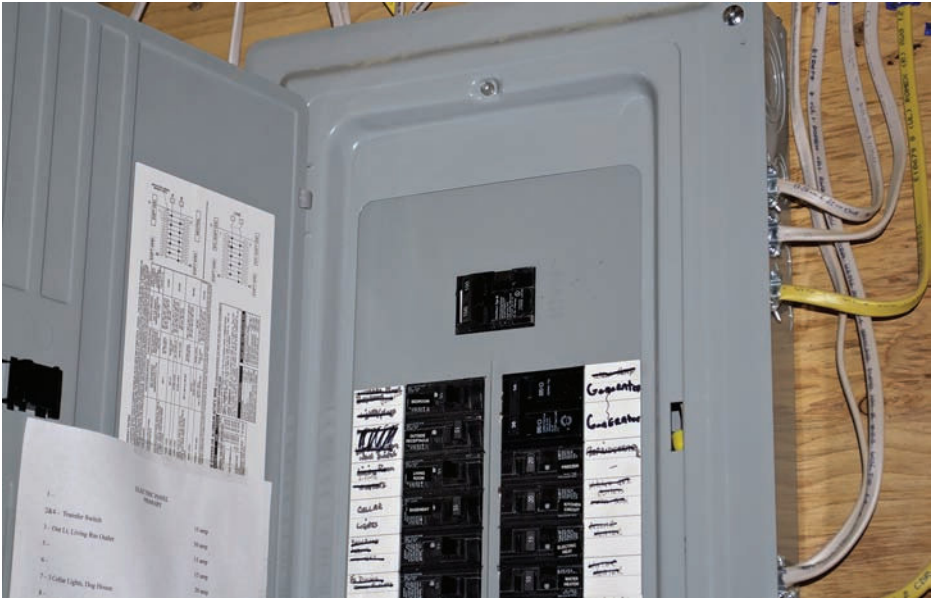
FIGURE G-12 The main disconnect is frequently located in the service-entrance panel.
