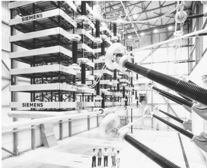
FIGURE 5.25 Valve hall of \pm 500 kV, 1000 MW long-distance HVDC converter station. (Photo courtesy Siemens.)
