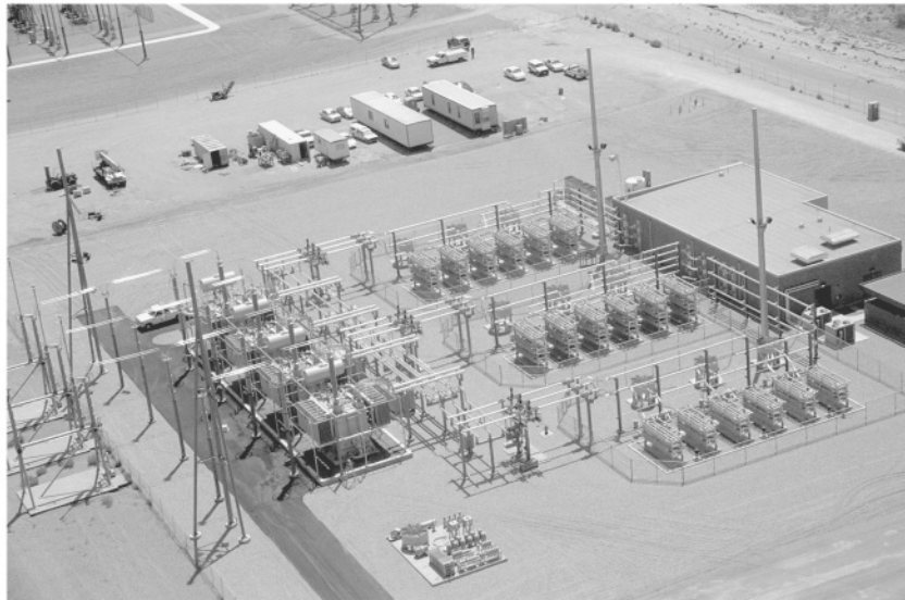
FIGURE 5.27 500 kV, 400 MVar SVC at Adelanto, California. (Photo courtesy Siemens.)
