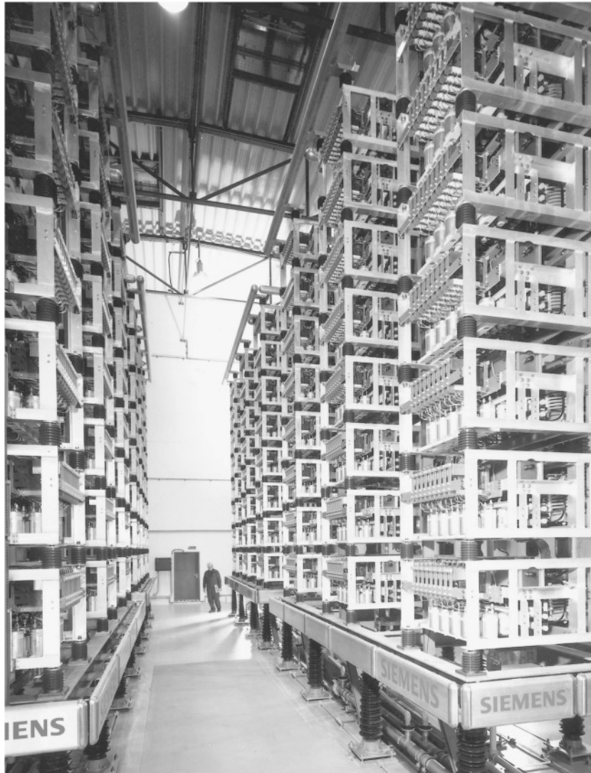
FIGURE 5.24 600 MW HVDC back-to-back converter valves. (Photo courtesy Siemens.)
