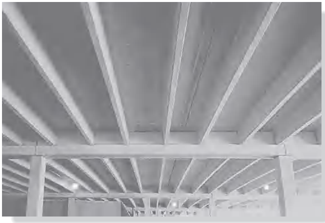
The simply supported girder of this concrete building frame was designed by first drawing its shear and moment diagrams.
