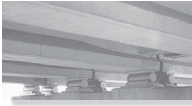
Rollers and associated bearing pads are used to support the prestressed concrete girders of a highway bridge.
