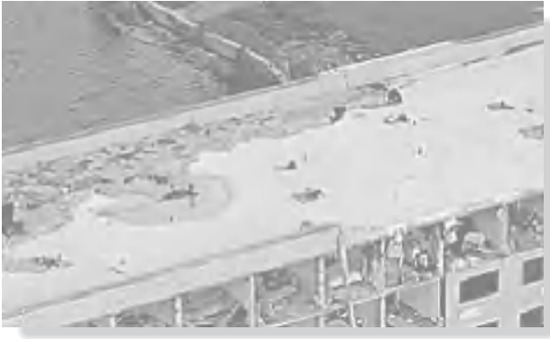
Hurricane winds caused this damage to a condominium in Miami, Florida.
