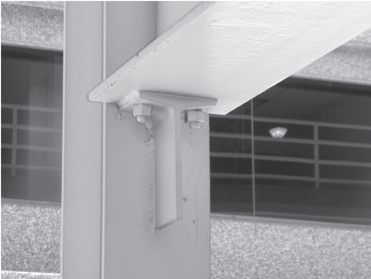
Fig. 11.33 Welded stiffened seat connection using the split I-section in a car parking structure in Bethesda, USA. (The bolts are erection bolts.)
