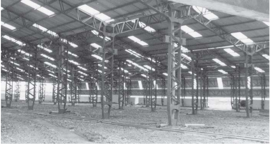
Built-up column in a portal frame, Mumbai (Note the stubs in the column, which carry a small crane).
