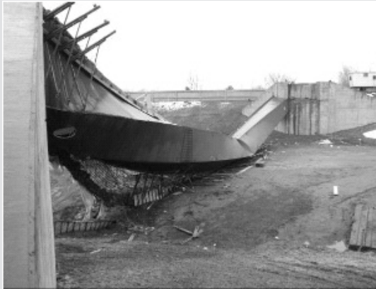
Fig. CS1 Cross-section of Marcy Bridge and the failure due to lateral-torsional buckling (source: Corr, et al, 2009)
