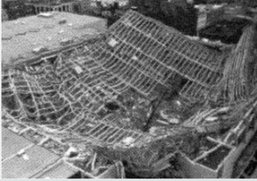
(c) View of the collapsed roof
