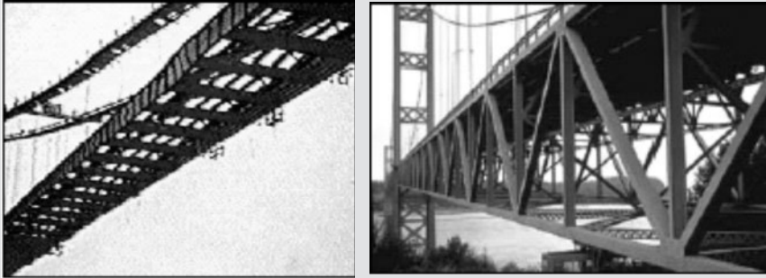
Fig. CS2 Solid I-beams in the deck of the original bridge and trussed deck of the reconstructed bridge ( www.failurebydesign.info )
