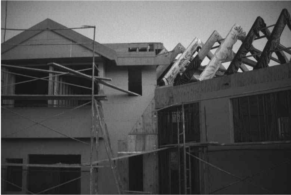
Figure A.7 Solar roof rafters in place preparing for the topping of large insulating R-control foam panels.
