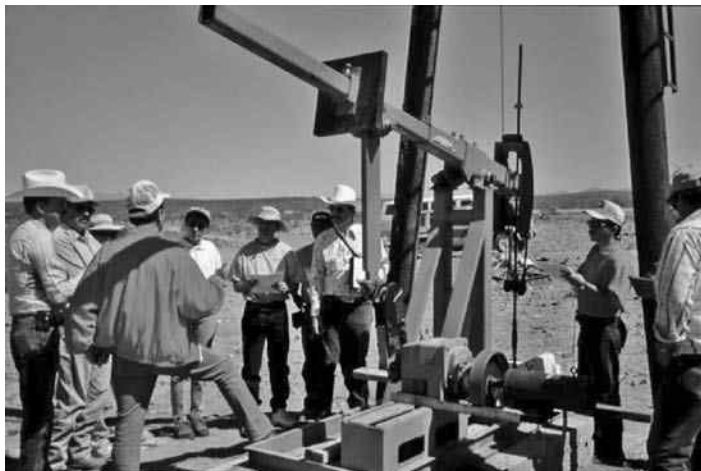
FIGURE 8.41 PV-powered surface jack pump in Chihuahua, Mexico, for a 170-meter deep well.
