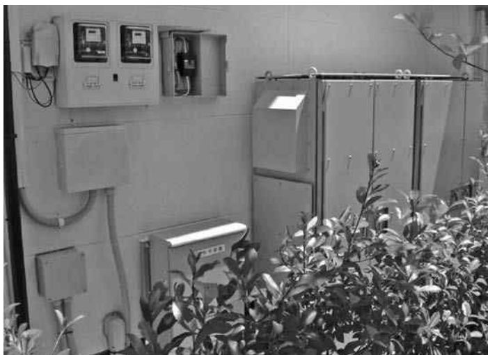
FIGURE 8.6 PV system grid inter-tie (note 2 meters) in Ohta City. Inverter and battery bank are housed in the large boxes on the right.
