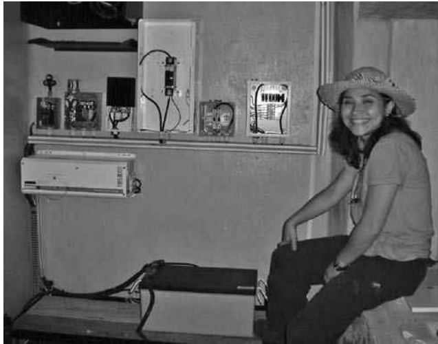
FIGURE 8.22 PV-powered COHCIT satellite telecenter with Internet connectivity using quality BOS components with master PV installer Ethel Enamorado in Sosoal, Lempira, Honduras.
