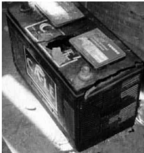
FIGURE 11.14 Exploded battery at Chiapas residence from ungrounded PV system hit by lightning.
