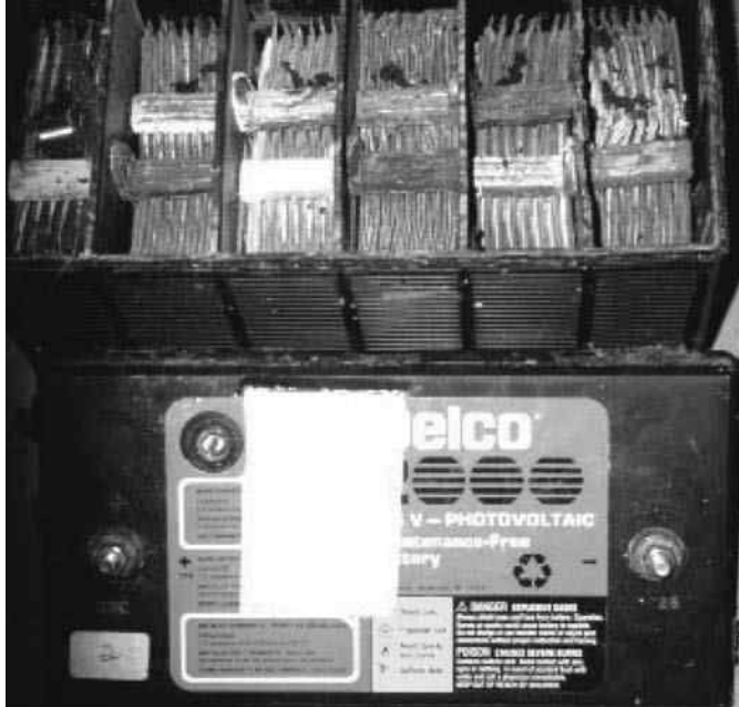
FIGURE 11.10 Excessive plate sulfation and buckling as a result of consistent undercharging of a battery in Ceara, Brazil, for a small residential PV home system.
