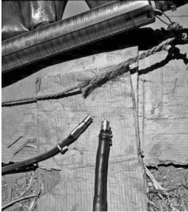
FIGURE 8.43 PV pump damaged cable splice where conductors have worn through from hauling the pump up and down on the pump cable rather than the security rope (Roatan, Honduras).
