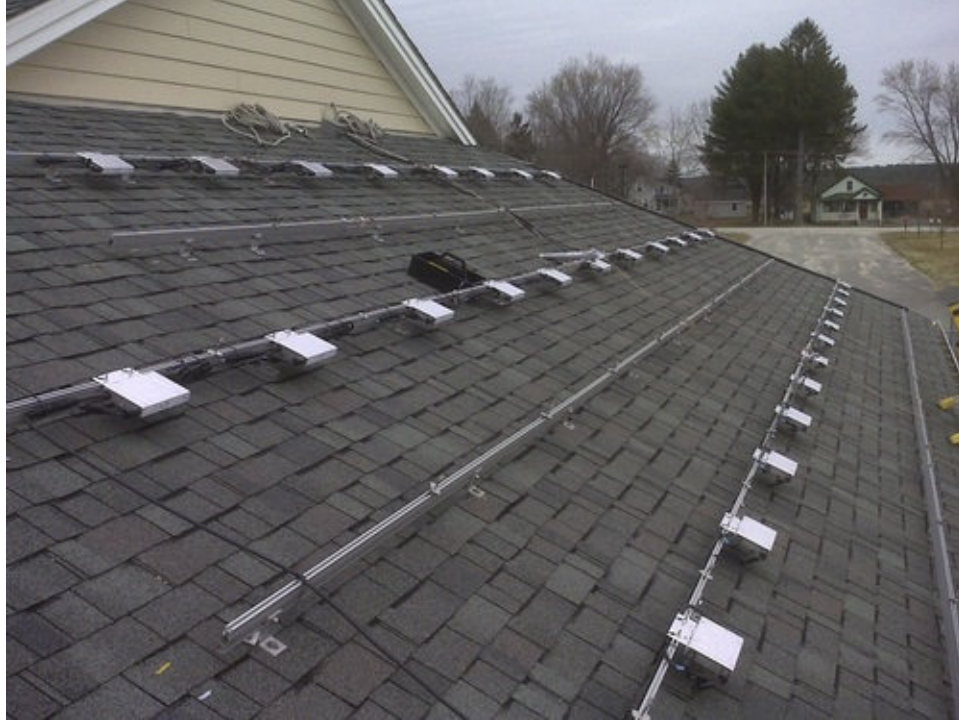
FIGURE 5.7 Microinverters and mounting system for PV modules. Photo courtesy of ReVision Energy Corp. (For color version of this figure, the reader is referred to the online version of this book.)
