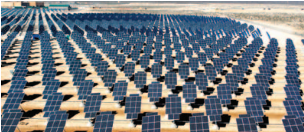
Photo 6.3 PV plants on Nellis Air Force Base, Nevada
