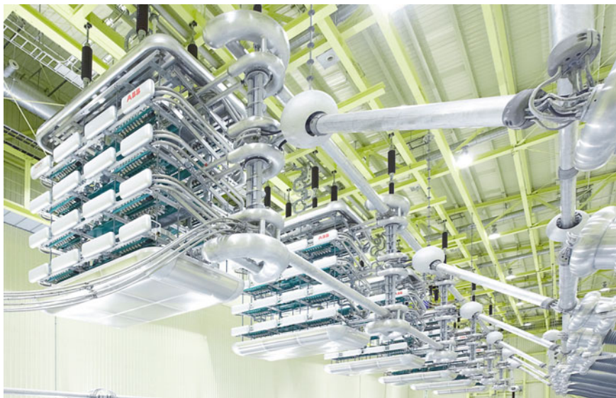
Fig. 3.46 Transformer bushings and valve towers of a \pm 800 kV converter station (Source ABB AG)
