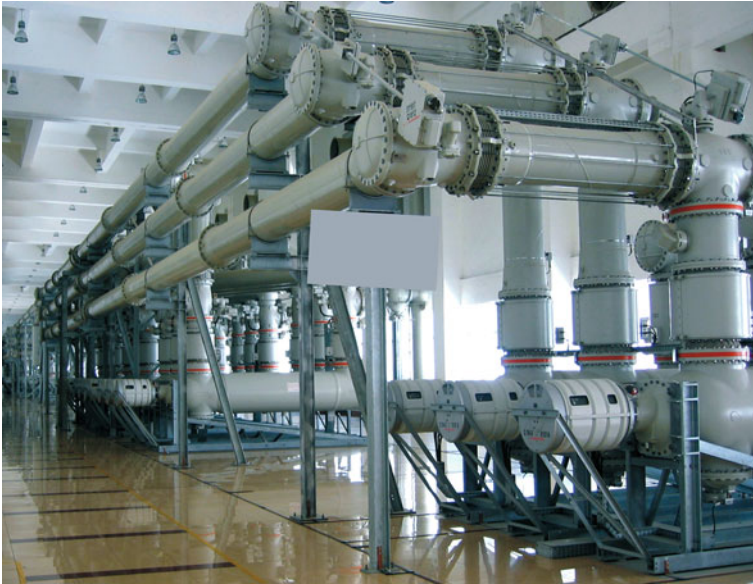
Fig. 3.13 A 550 kV SF 6 gas insulated switch plant (Source ABB AG, Type ELK_3_S9)
