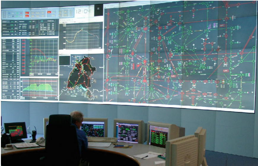
Fig. 3.37 View of a transmission system dispatching center (Source Siemens AG)
