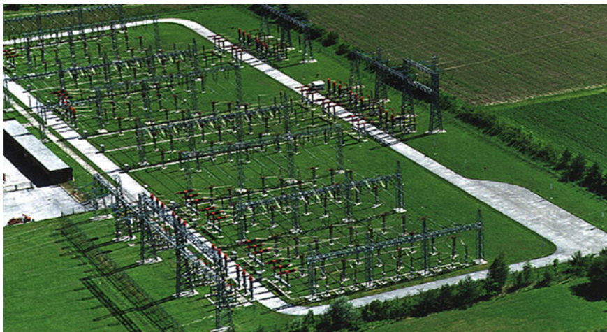
Fig. 3.1 View of an open air EHV/HV substation (Source Siemens AG)
