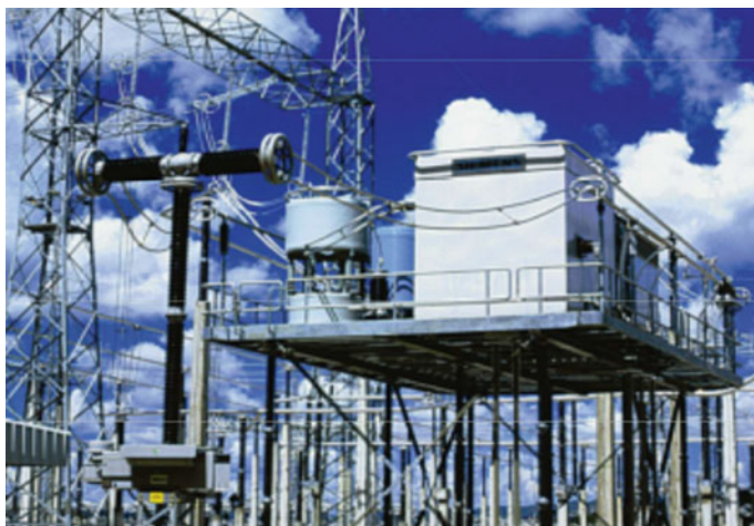
Fig. 3.54 TCSC installation of a 500 kV line ( Source Siemens AG )
