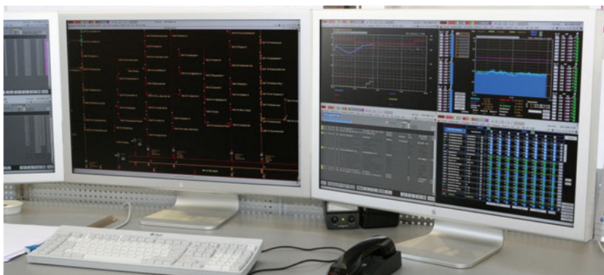
Fig. 4.36 The workplace for electric network operations in a DCC. Source HSE AG
