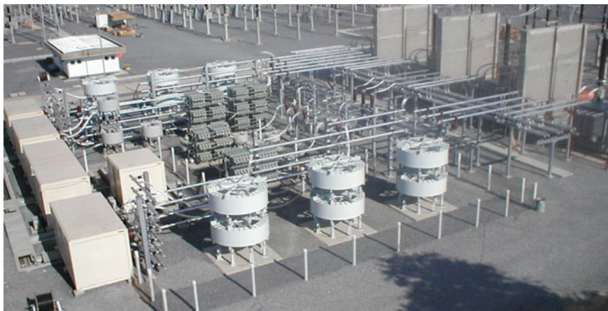
Fig. 3.53 SVC plant \pm 250 Mvar ( Source Siemens AG )
