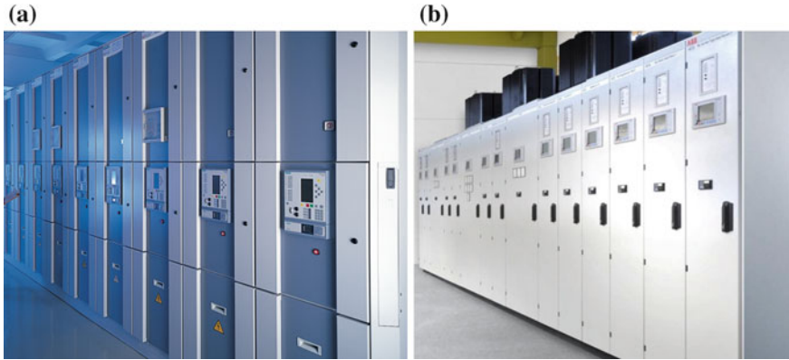
Fig. 4.28 Advanced switch bay cubicles 20 kV with local control by a combined device for protection and control. Sources a Siemens AG, b ABB AG
