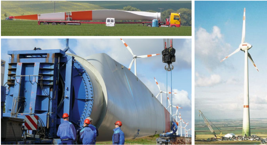
Fig. 2.4 Erection of a wind power plant 6.5 MW: rotor length 60 m (Source Regenerativ-Kraftwerk Harz GmbH and Co.KG. [9])
