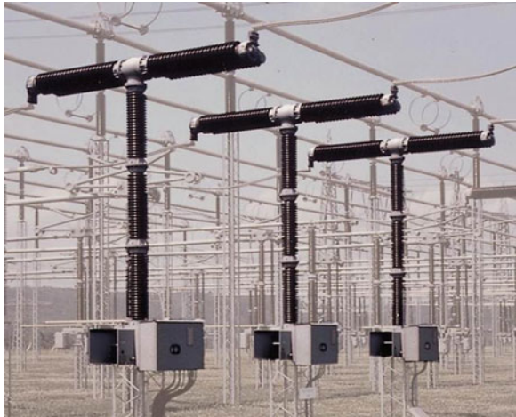
Fig. 3.10 SF 6 circuit breaker in a 400 kV substation (Source Siemens AG)
