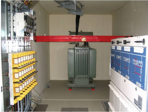
Fig. 4.9 Ring main terminal with the 400 V distribution panel. Source HSE AG
