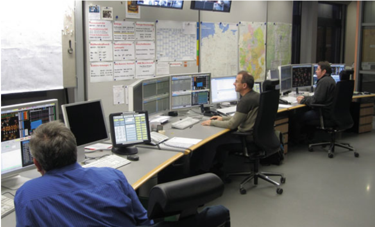
Fig. 4.35 Multi-utility DCC with three work separate workplaces for electricity, gas and heat. Source HSE AG
