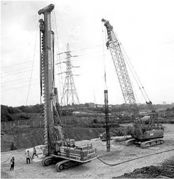
Figure 3.33 Installation of CFA piles in chalk with crane handling reinforcement cage (courtesy Cementation Foundations Skanska).
