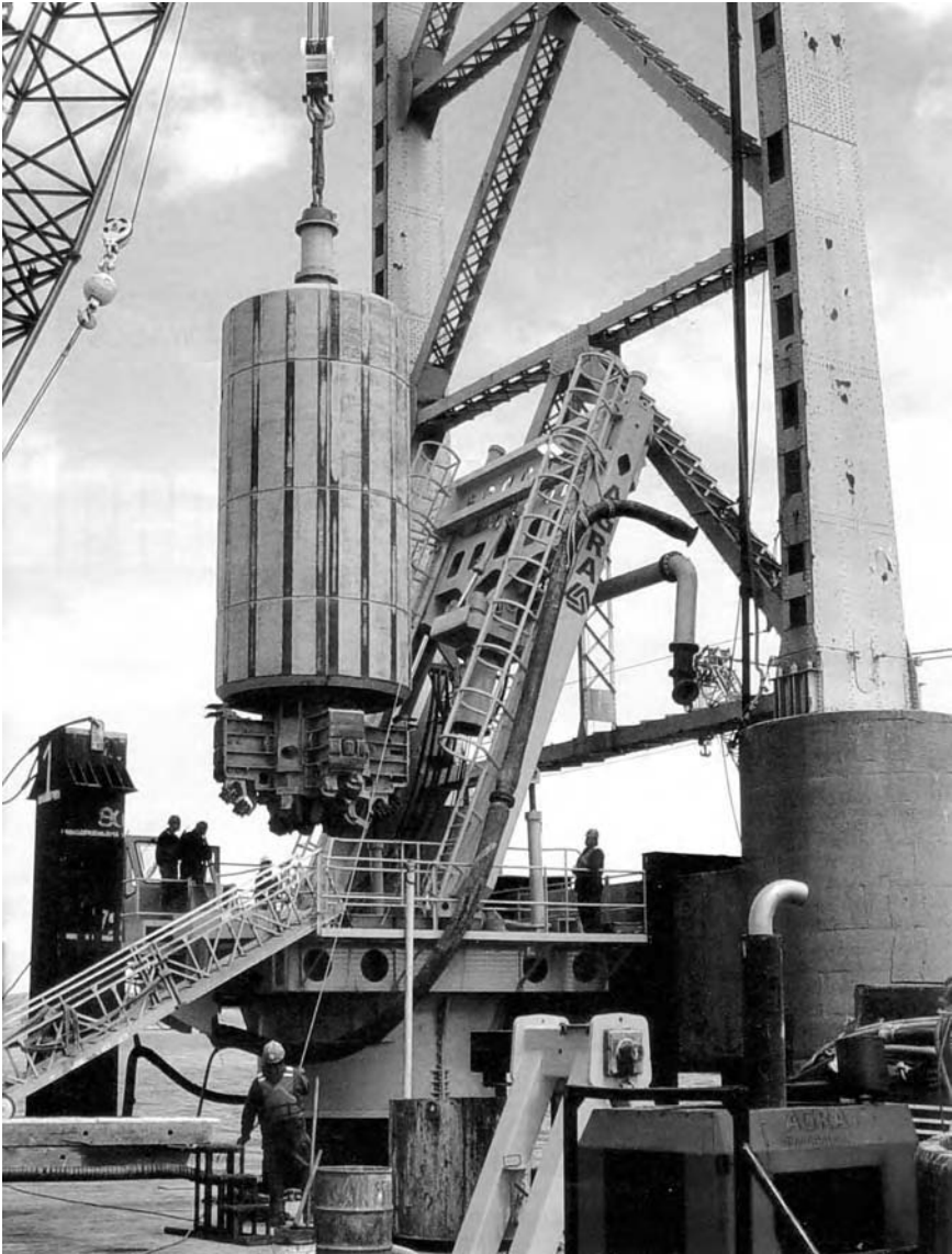
Figure 3.36 Pile top rig drilling 3.8 m dia piles for foundation strengthening to the Richmond-San Raphael bridge, California (courtesy Seacore Ltd).
