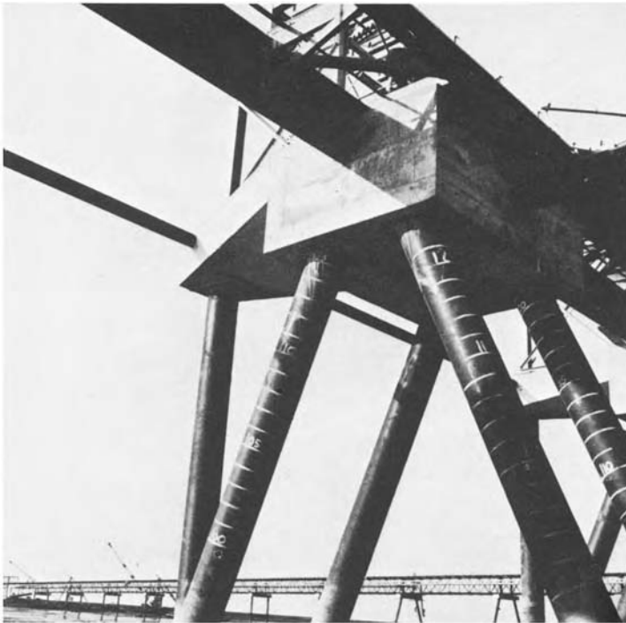
Figure 8.2 Raking and vertical piles used to restrain berthing forces in bulk handling jetty.
