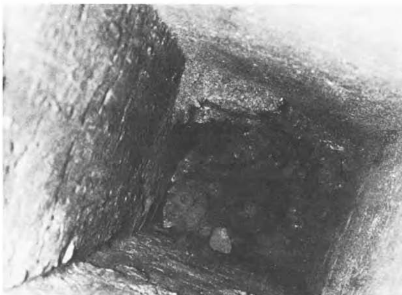
Figure 10.1 Decay of timber piles above groundwater level (Crown copyright reserved) (a) Cavities left by complete decay of piles and timber capping sills (b) View down cavity left in clay after complete decay of timber pile.
