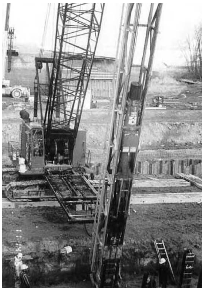
Figure 3.15 Delmag D30–20 diesel hammer on American style leaders with helmet for driving steel H-piles.
