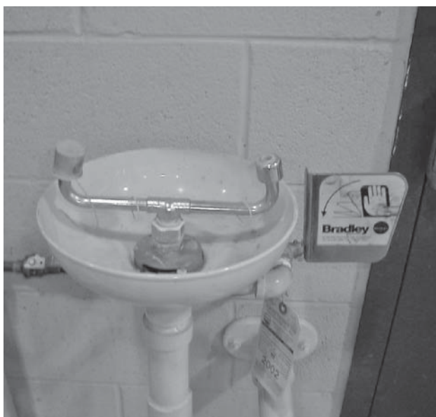
Figure 1-4 Emergency eye wash station.
