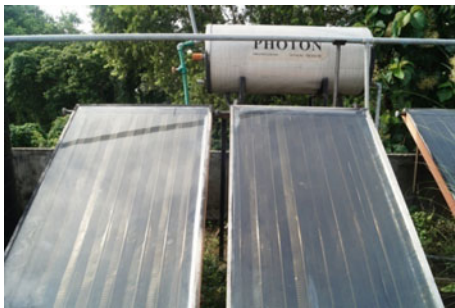
Solar water heater
