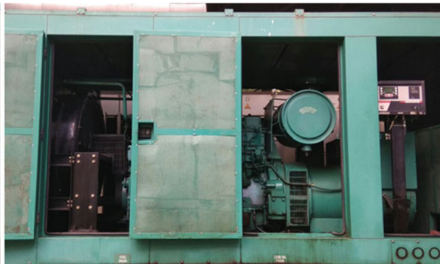
Diesel engine generator
