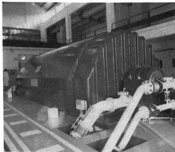
Figure 8.5 View of LAPEM's Test Generator (Courtesy of LAPEM, Irapuato, Gto. Mexico)
